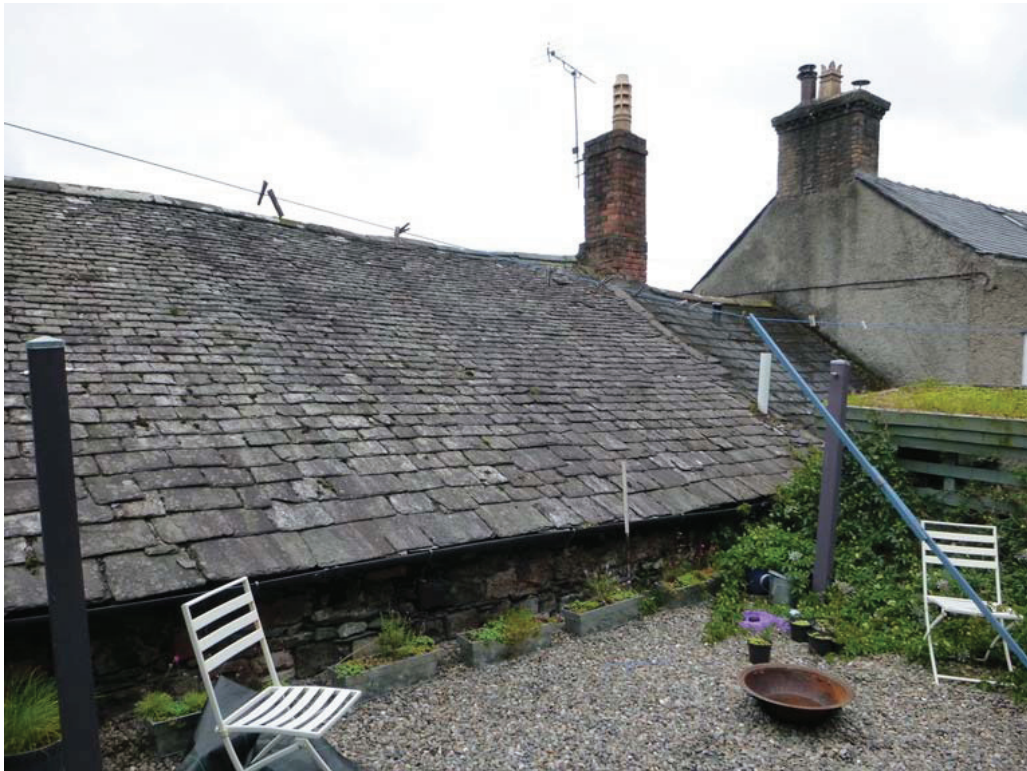
Plate 17: The south end of the west external elevation, viewed from the north-west
