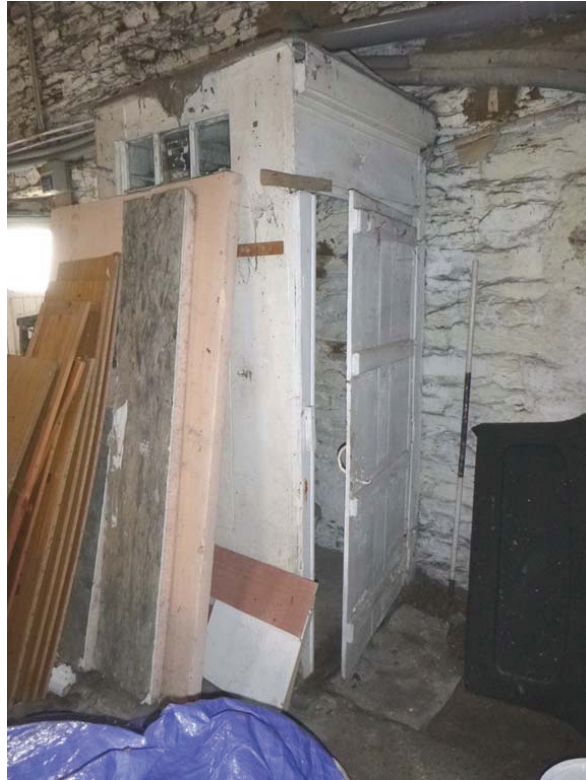
Plate 32: The partition walls forming a toilet against the south internal elevation, viewed from the north-west
