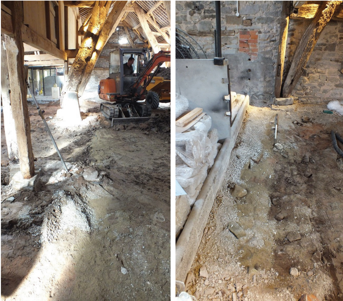
Plate 114 (left): View along the trench for the electric cables connecting the recessed flood lights along the west side of Room 2
