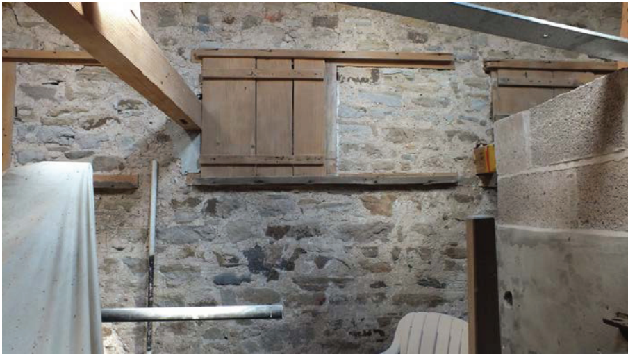
Plate 100: Opening with overlong sill and lintel in the east elevation of Room 4
