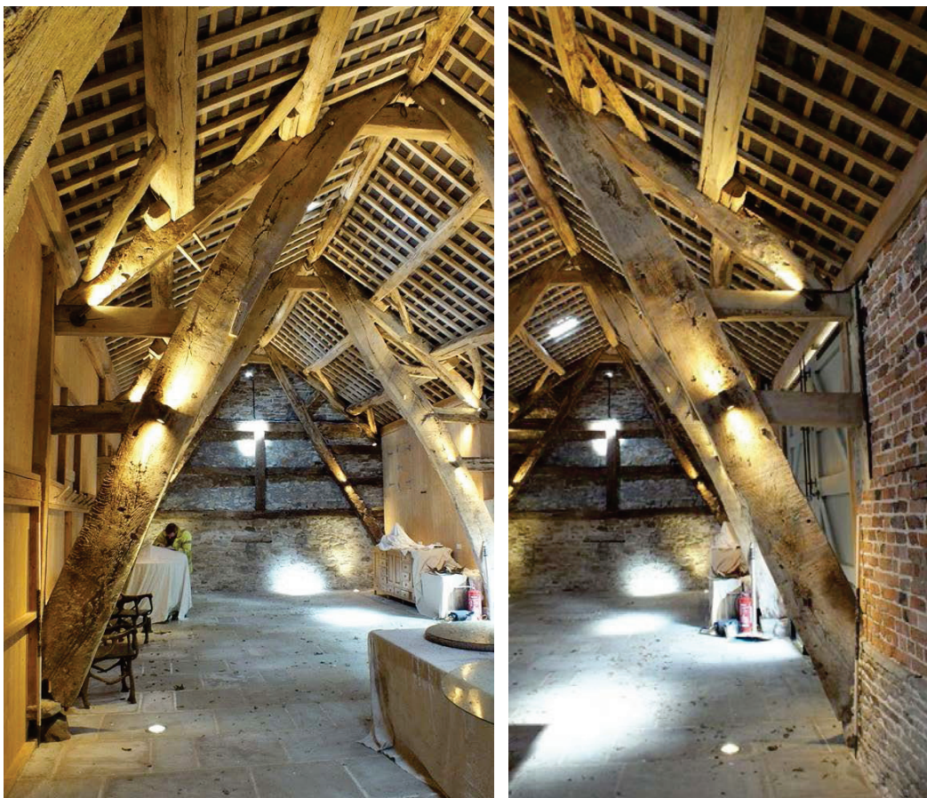
Plate 45 (left): The west side of the south face of Truss 3, Room 2 Plate 46 (right): The east side of the south face of Truss 3, Room 2
