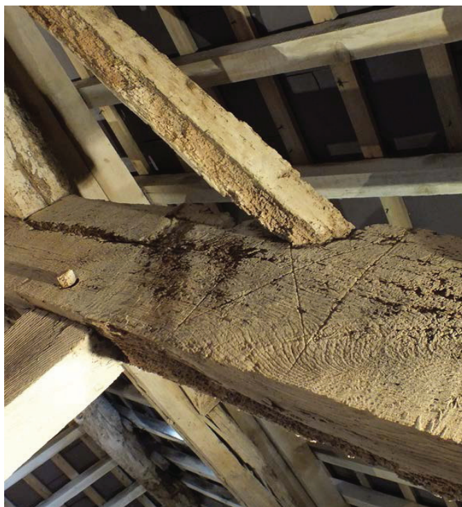
Plate 59: Levelling mark on west side of the north face of Truss 5, Room 2
