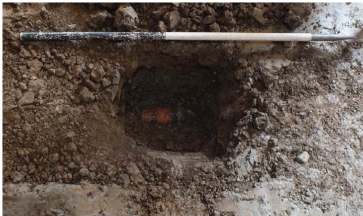
Plate 113: Drain pipe wrapped in plastic at the base of the wide drain cut in Room 2
