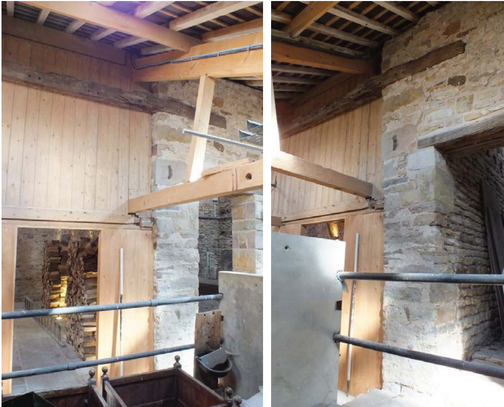
Plate 97 (left): Wall plate above the planking and stone sections on the east elevation of Room 4
