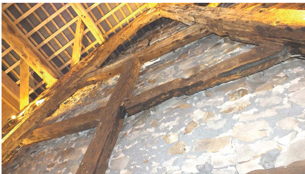
Plate 32: The underside of Truss 1, Room 2
