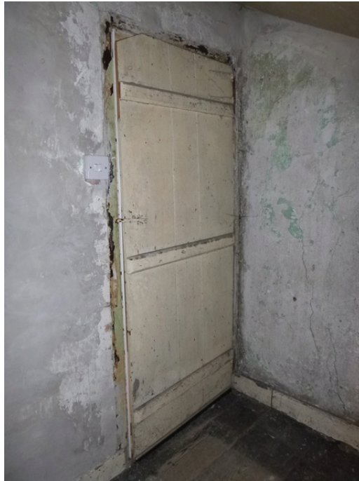
Plate 85: the doorway on the east side of Room F11, viewed from the north-west
