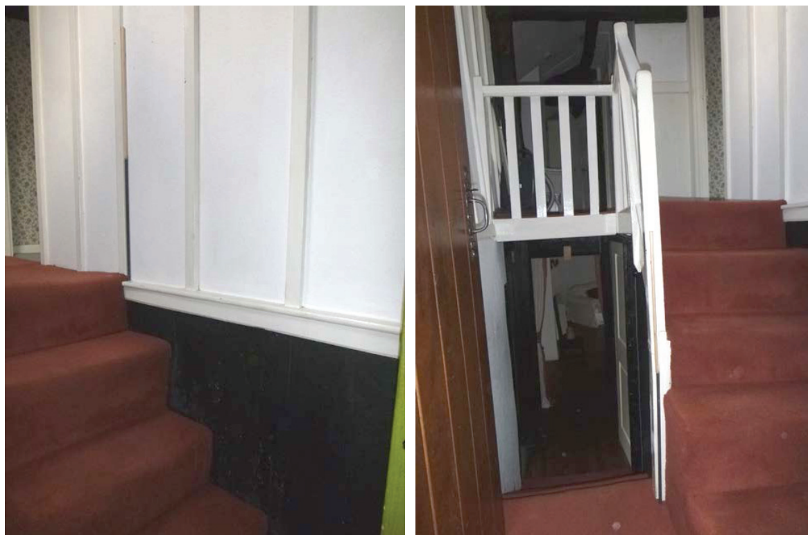
Plate 36 (left): the plank and mutin wall on the south side of Room G4, viewed from the north-east
