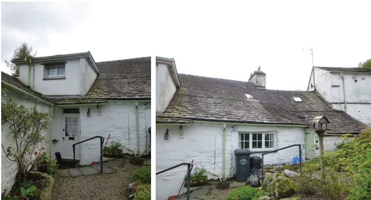
Plate 11 (left): the dormer window on the west side of the central part of the north external elevation, viewed from the north-west
