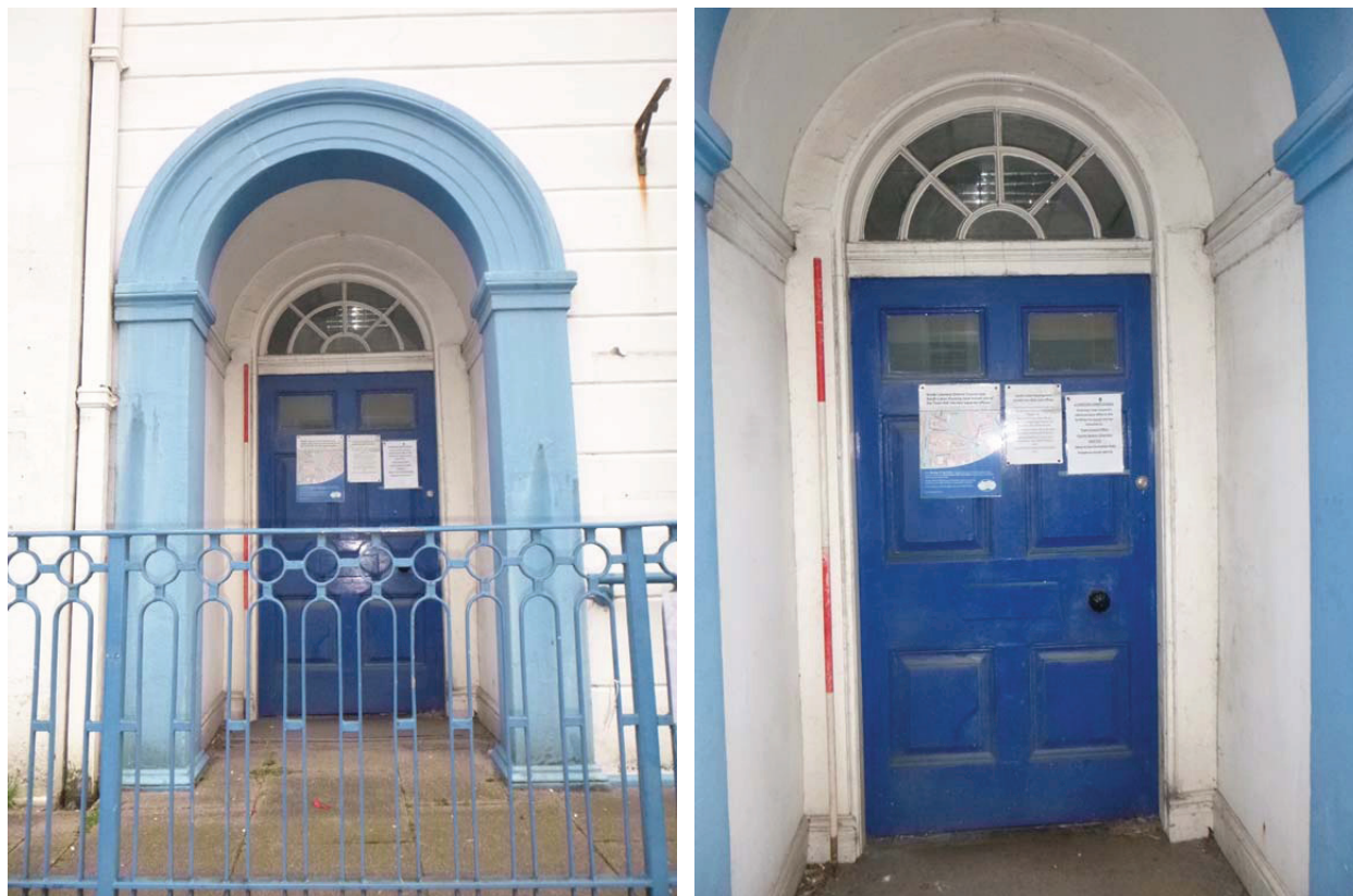
Plate 88 (left): The southern doorway in the west external elevation, viewed from the west
