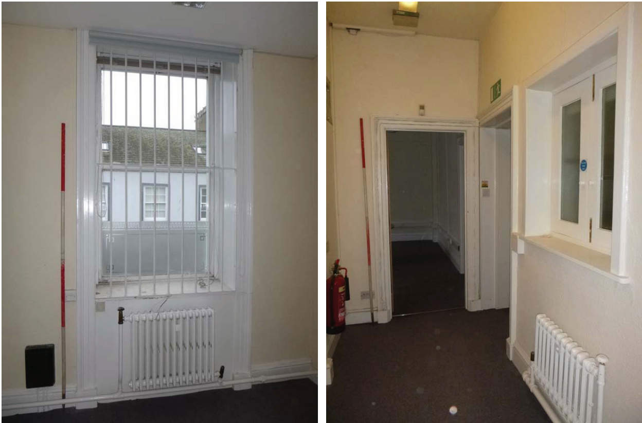
Plate 173 (left): Window in the west elevation of Room F2, viewed from the east
