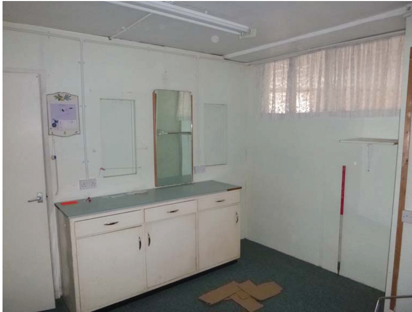
Plate 166: General view of the north and east elevations of Room G24, viewed from the south-west
