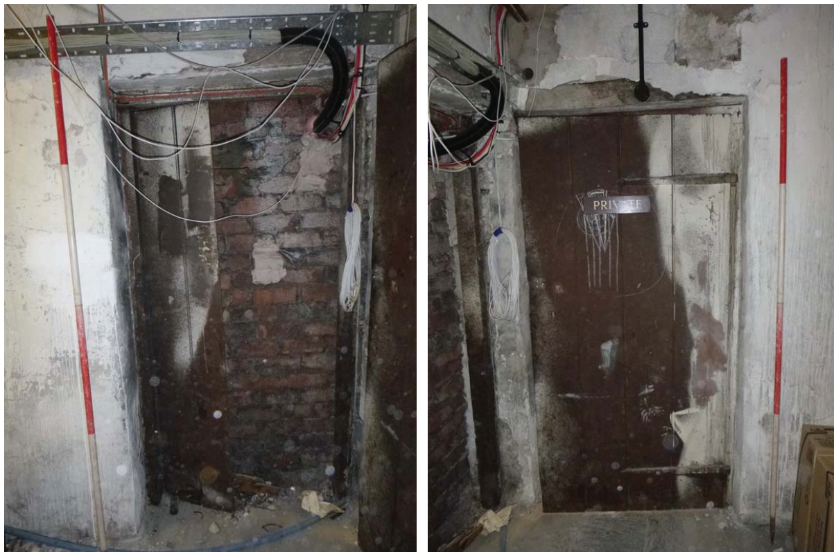
Plate 115 (left): The blocked doorway to the south in Room B8, viewed from the north
