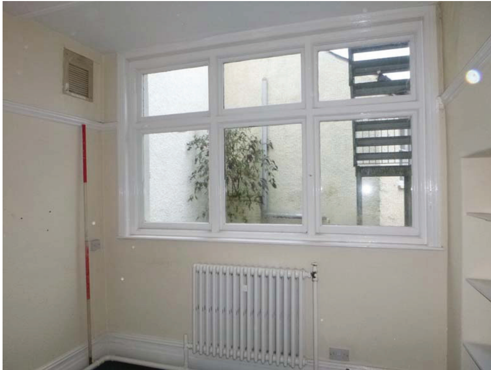
Plate 151: The window in the east elevation of Room G11, viewed from the south-west
