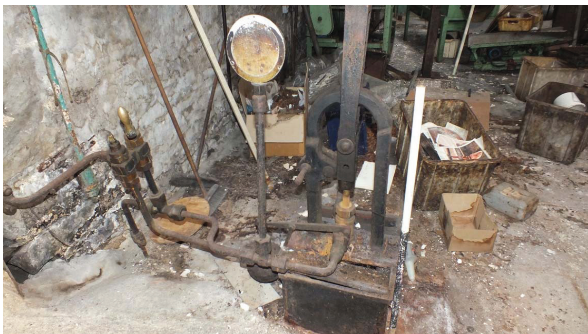
Plate 41: Extant pressure gauge on the north-west side of Room G6
