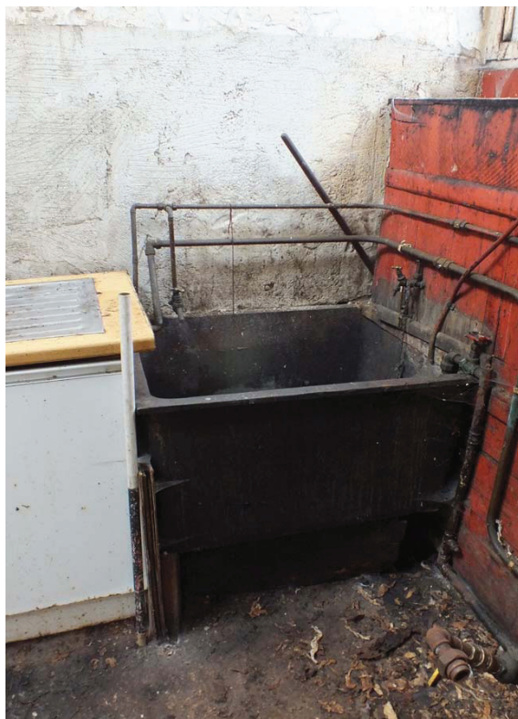
Plate 55: Iron tank on the east side of the north elevation, Room F13
