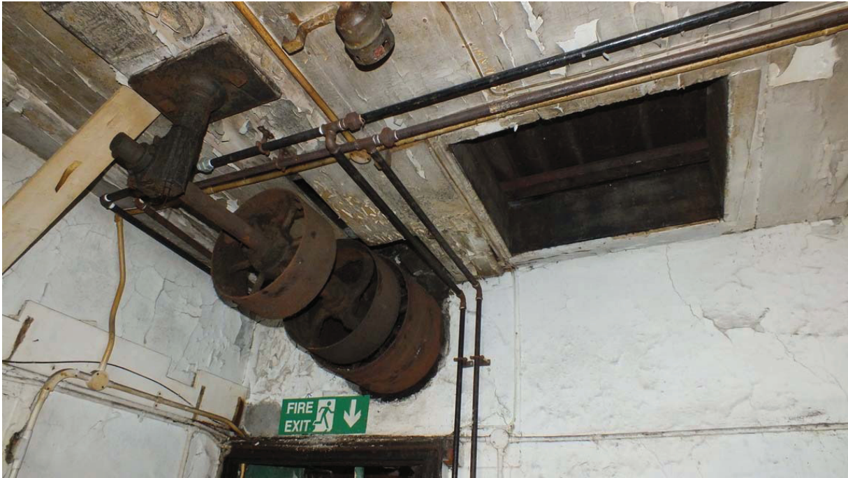
Plate 37: Drive shaft and adjacent hatch on the south-west side of the ceiling of Room G4
