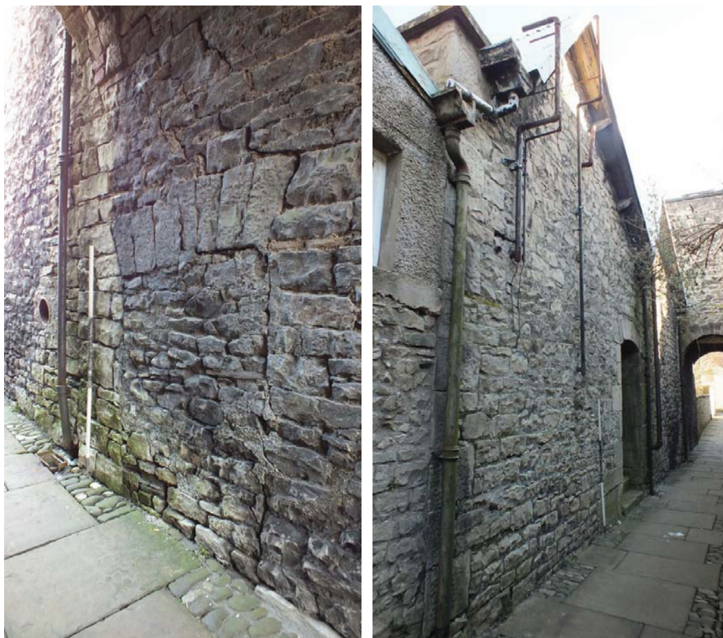
Plate 22 (left): East side of the south external elevation, showing the blocked opening
