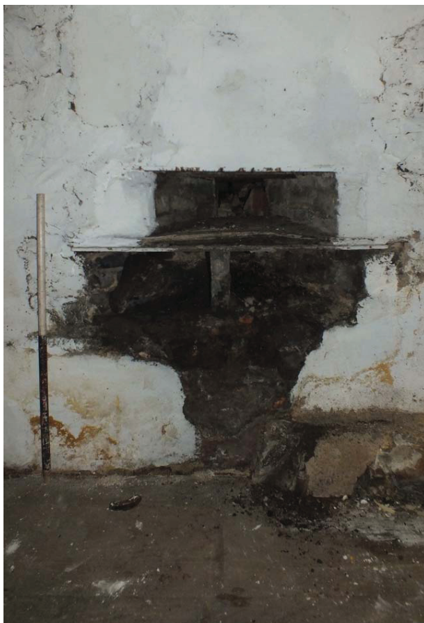
Plate 26: Aperture in the north elevation of the southern room of Cellar A
