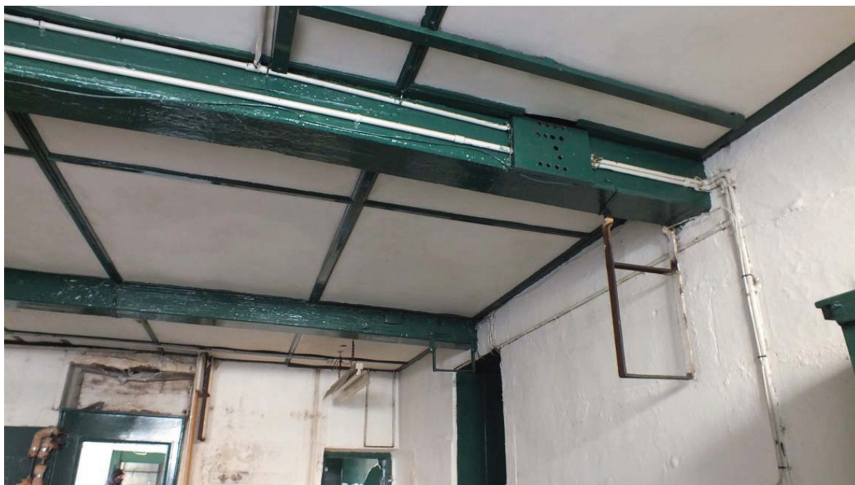
Plate 32: Iron loops attached to the beams along the east and south sides of Room G2
