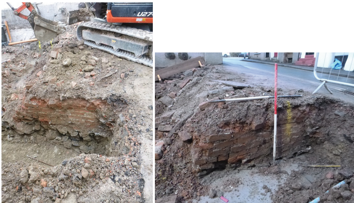
Plate 26 (left): East-facing elevation of wall 108 along the east-facing section of the north end of the east foundation trench, immediately prior to concrete being poured, taken from the east
