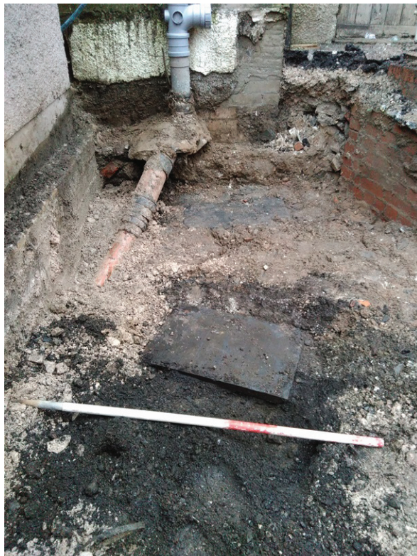
Plate 23: The furthest extent west of flag surface 109 (centre rear, with pipe to left), and polished stone flag within black bedding layer 112, taken from the east
