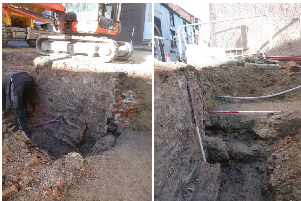
Plate 28 (left): Section of wall 108 following removal of the wall, showing rubble and large foundation boulders, taken from the south
