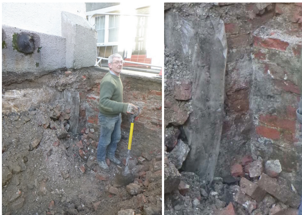
Plate 39 (left): Working shot showing the junction of wall 116 and wall 119, taken from the south-east Plate 40 (right): Close up of junction of wall 116 and wall 119, showing wall 119 butting against wall 116, following removal of top few courses of bricks from wall 119
