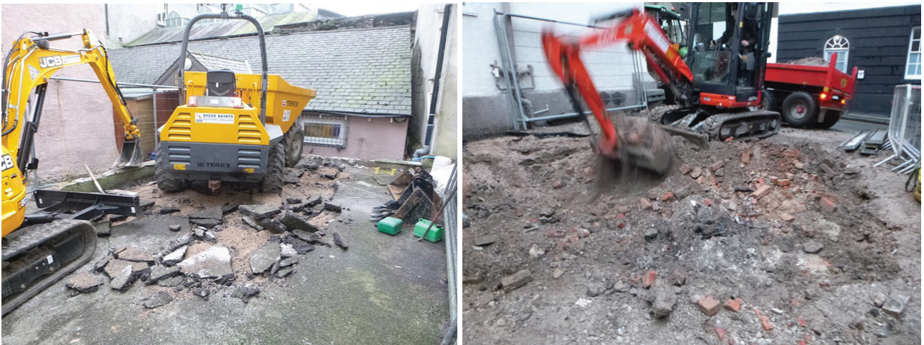
Plate 1 (left): Breaking up the tarmac at the start of the watching brief, facing the kitchen on the south of the site
