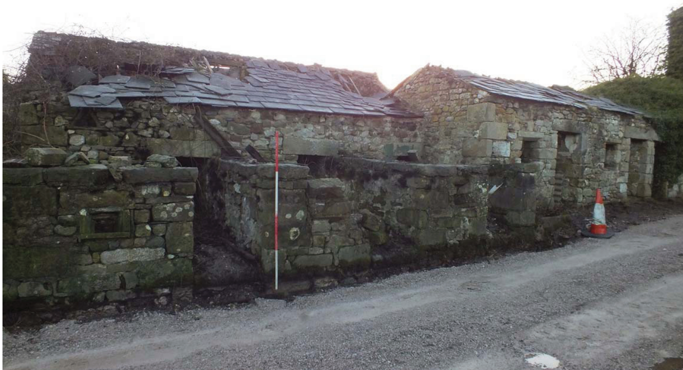
Plate 30: The north end of the west external elevation of the north/south block, showing its relationship to the south end
