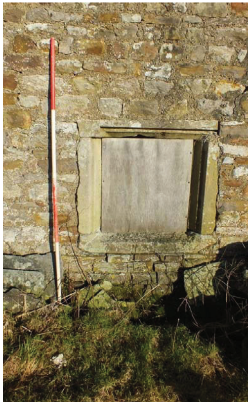
Plate 24: Window with moulded surround on the east side of the south external elevation of the main block
