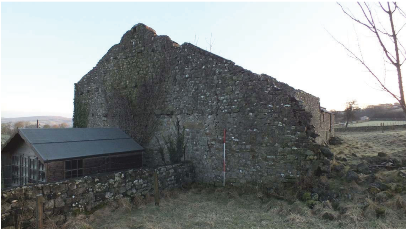
Plate 27: The south side of the west external elevation of the main block
