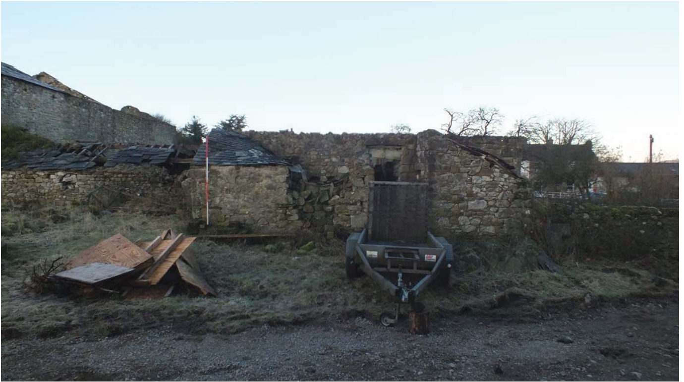
Plate 33: The north end of the east external elevation of the north/south block
