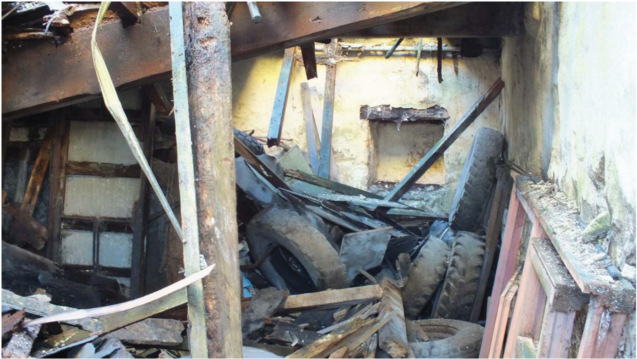
Plate 42: The alcove on the west side of the south elevation in Room G4
