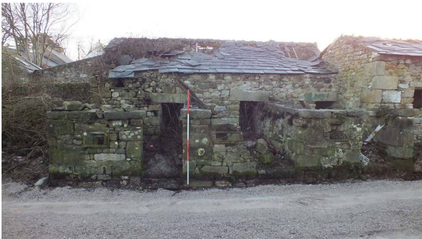
Plate 31: The north end of the west external elevation of the north/south block
