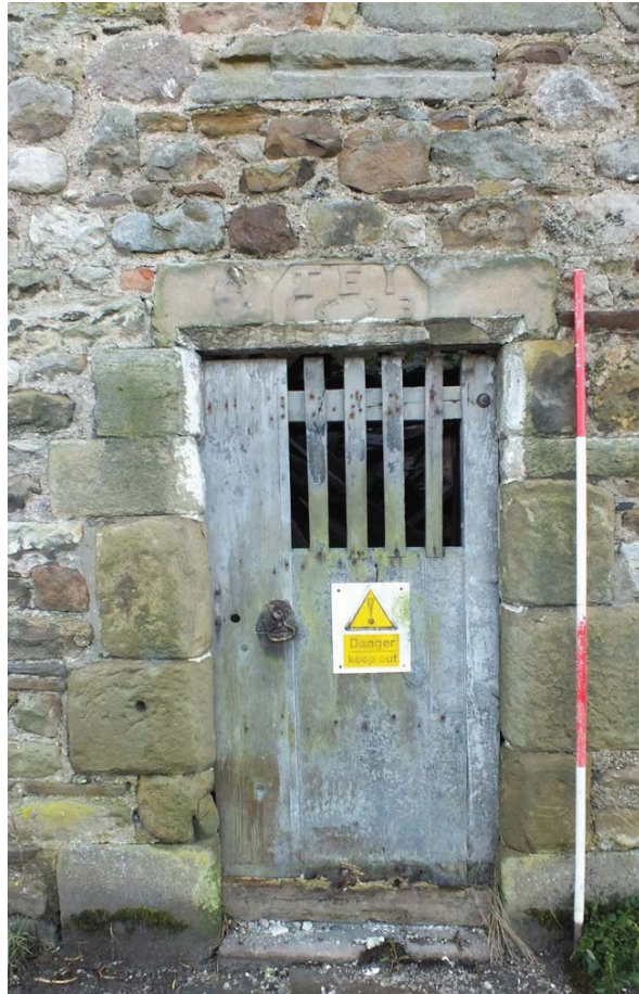
Plate 14: Doorway in the north external elevation of the main block with the datestone 'TEI 1693' and reused stone above
