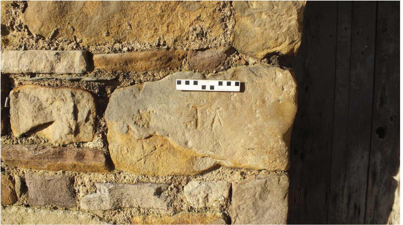
Plate 23: Graffiti 'JA' carved into a quoin in the return at the east end of the south external elevation of the main block
