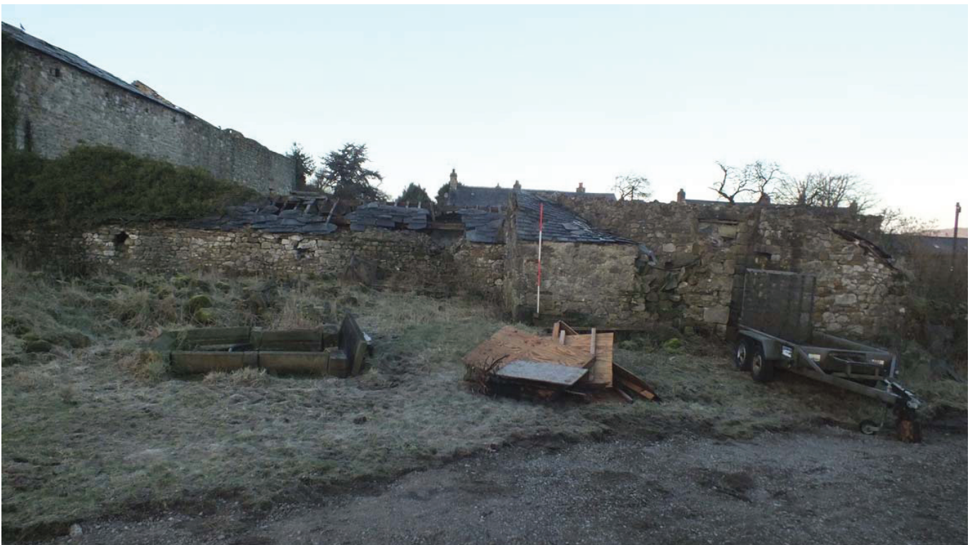
Plate 34: The south end of the east external elevation of the north/south block
