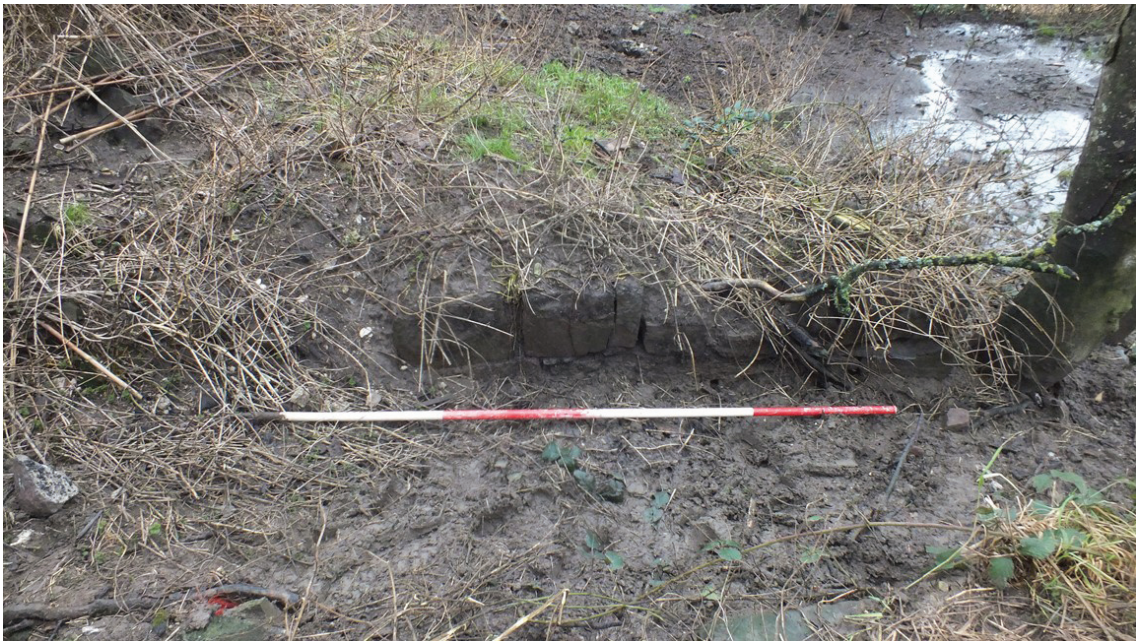
Plate 16: East wall elevation of the wheel pit to the west side of Building 2, viewed from the east
