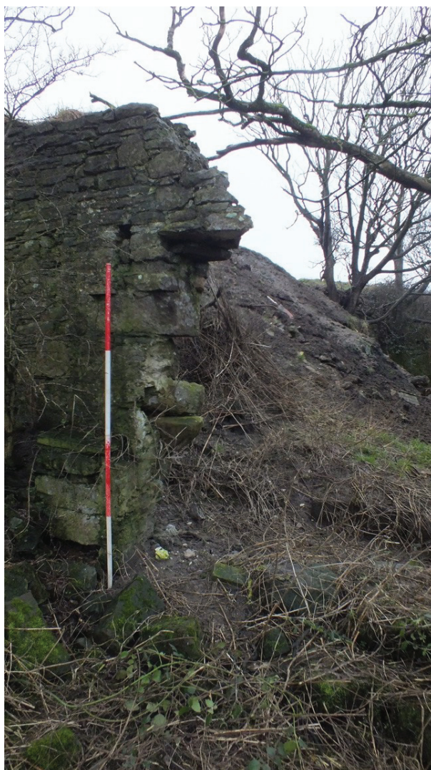
Plate 18: North end of the east elevation of Building 2 showing the opening(s), viewed from the north-east
