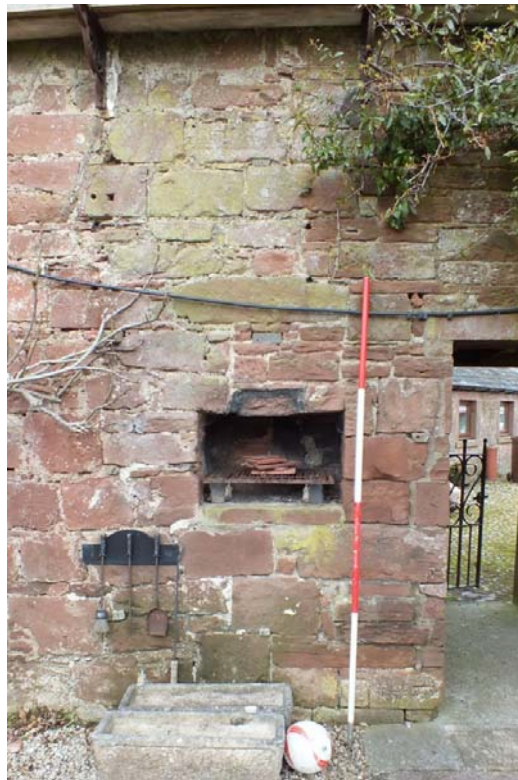
Plate 12: Fireplace built into the east end of the south external elevation, viewed from the south
