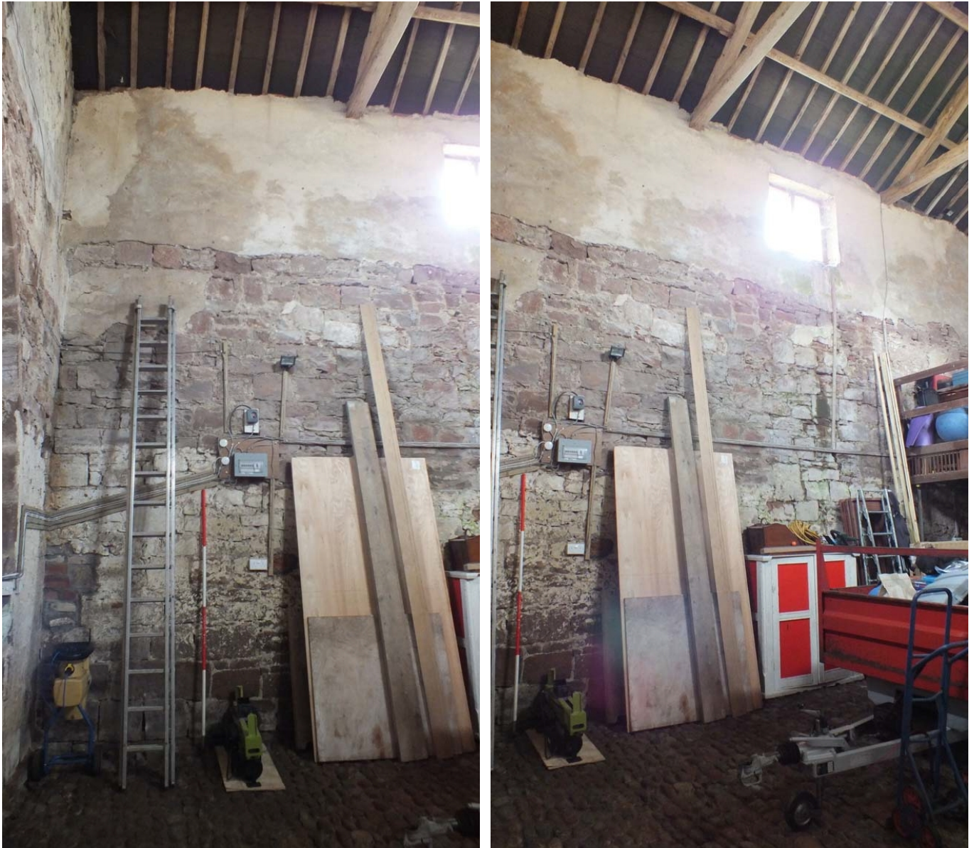
Plate 24 (left): The east side of the south internal elevation showing the brick rebuild, viewed from the north
