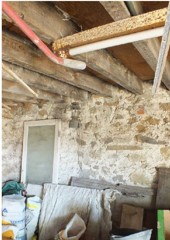
Plate 61: Red brick infill in the north-west internal elevation of Barn 3 below the hayloft
