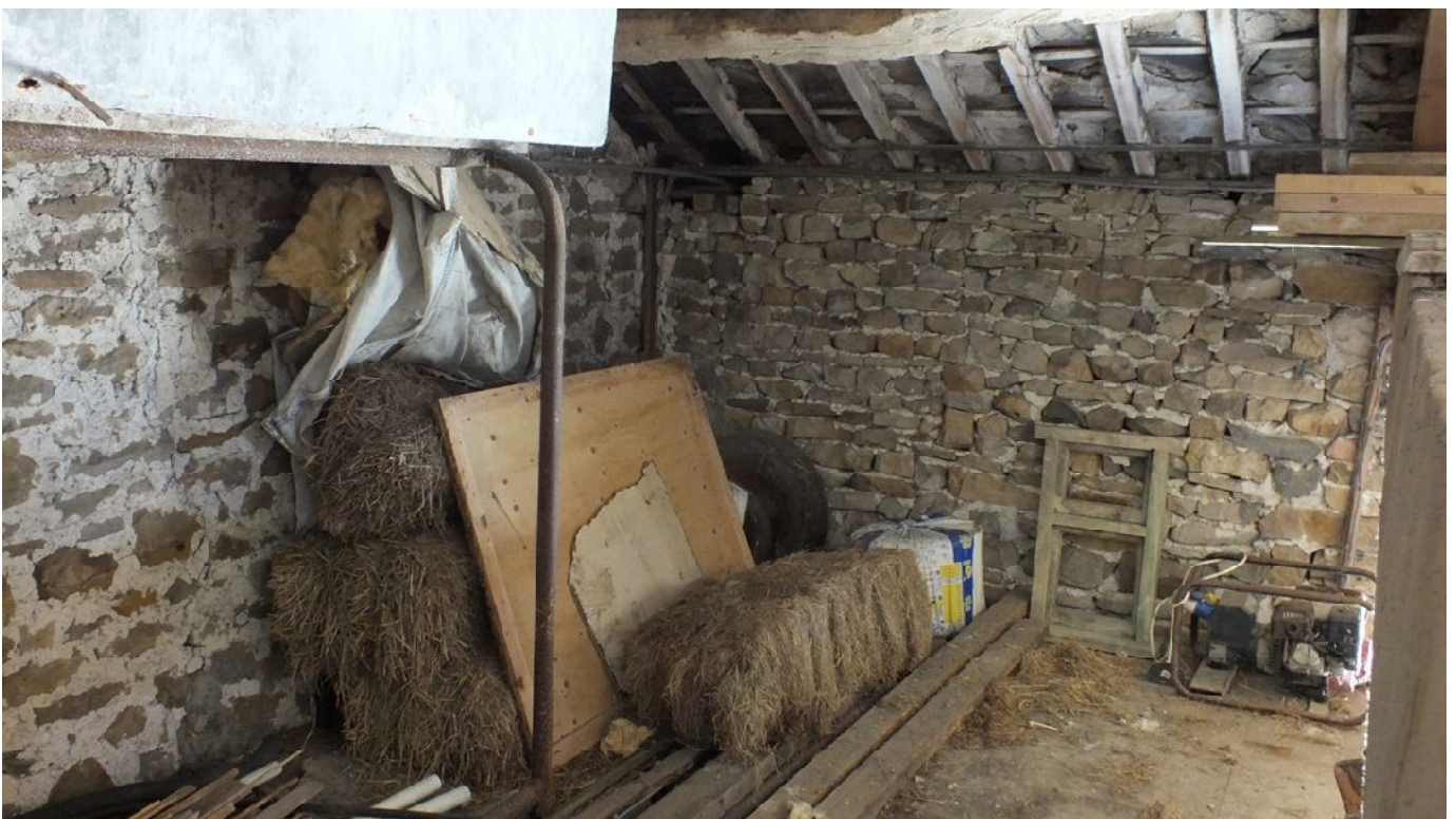
Plate 65: The north-west end of the north-east internal elevation of Barn 3 at the upper floor level
