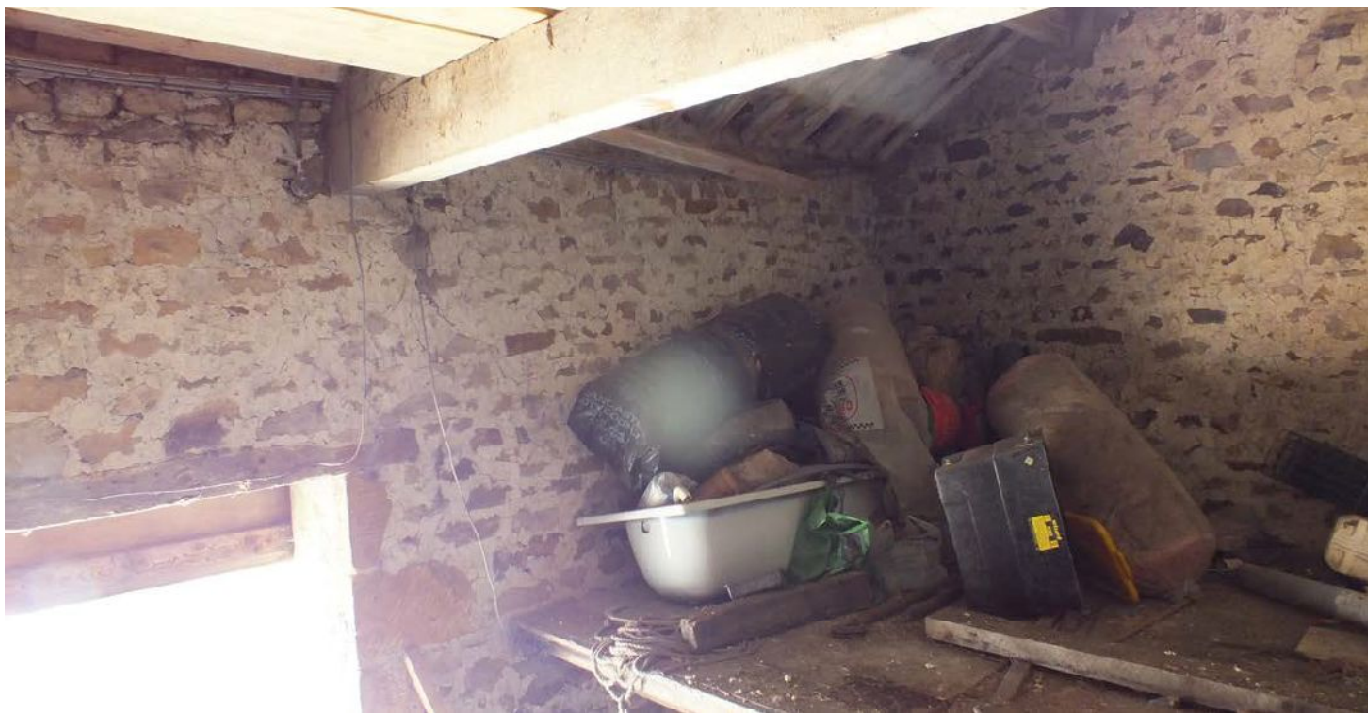
Plate 66: The south-east end of the north-east internal elevation of Barn 3 at the upper floor level
