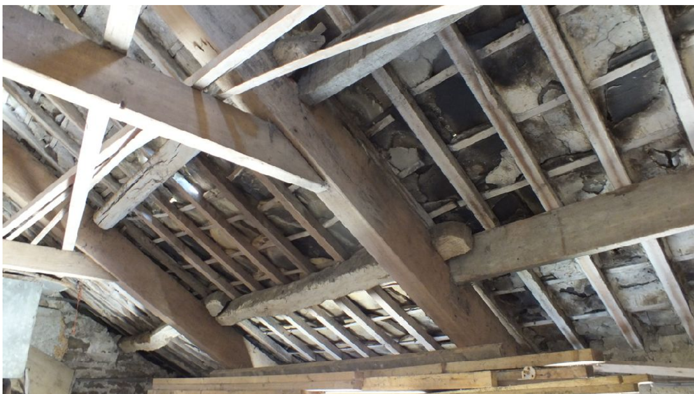
Plate 54: Old purlins above the wagon door and at the north end to the north-east side of Barn 3
