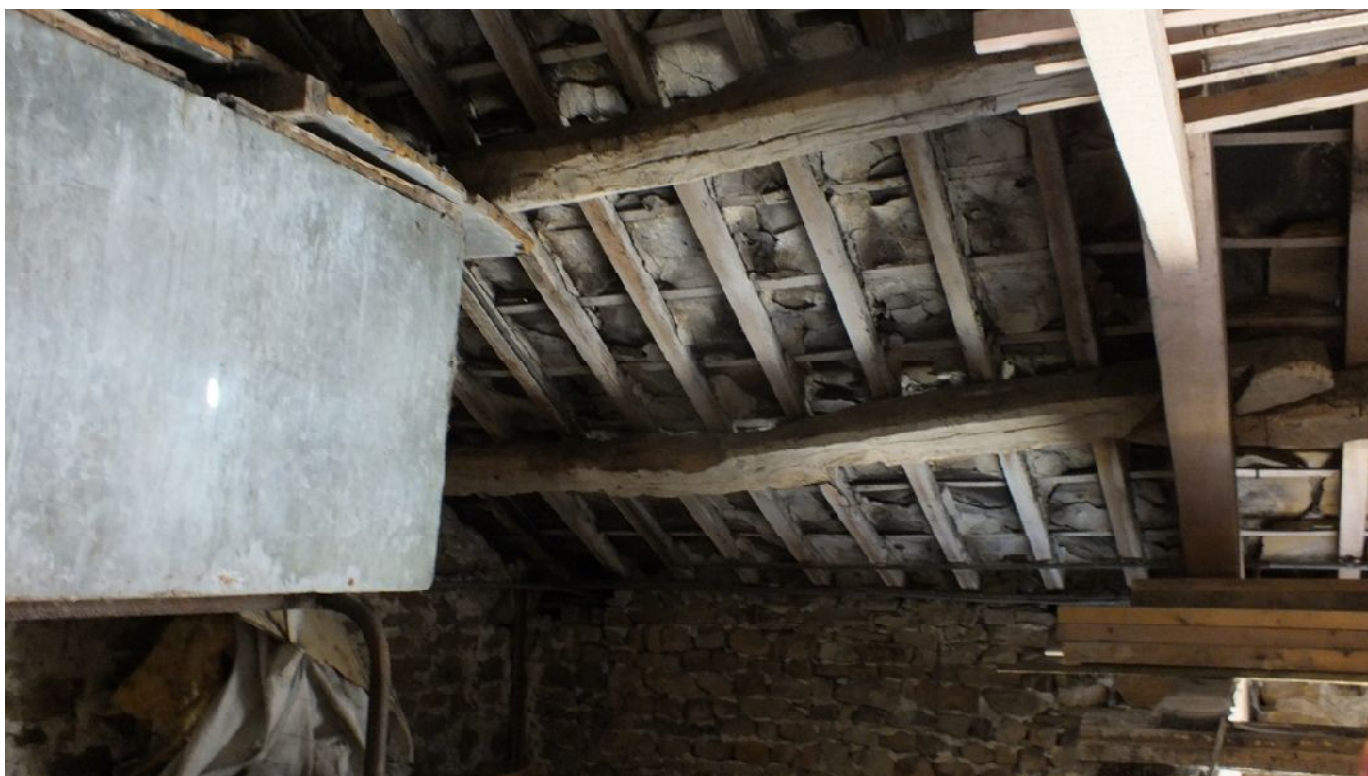
Plate 53: Old purlins in the north corner to the north-east side of Barn 3
