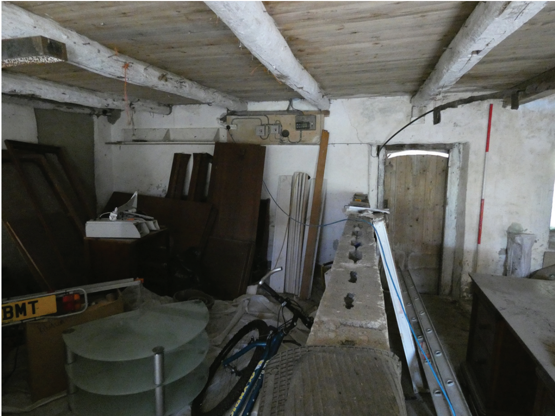
Plate 28: Partition wall between G1 and G2 and the south-west end of the north-west elevation
