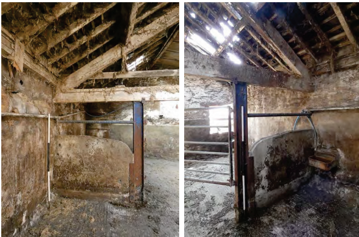
Plate 26 (left): Stall against the south-west elevation of Room G4, viewed from the south-east
