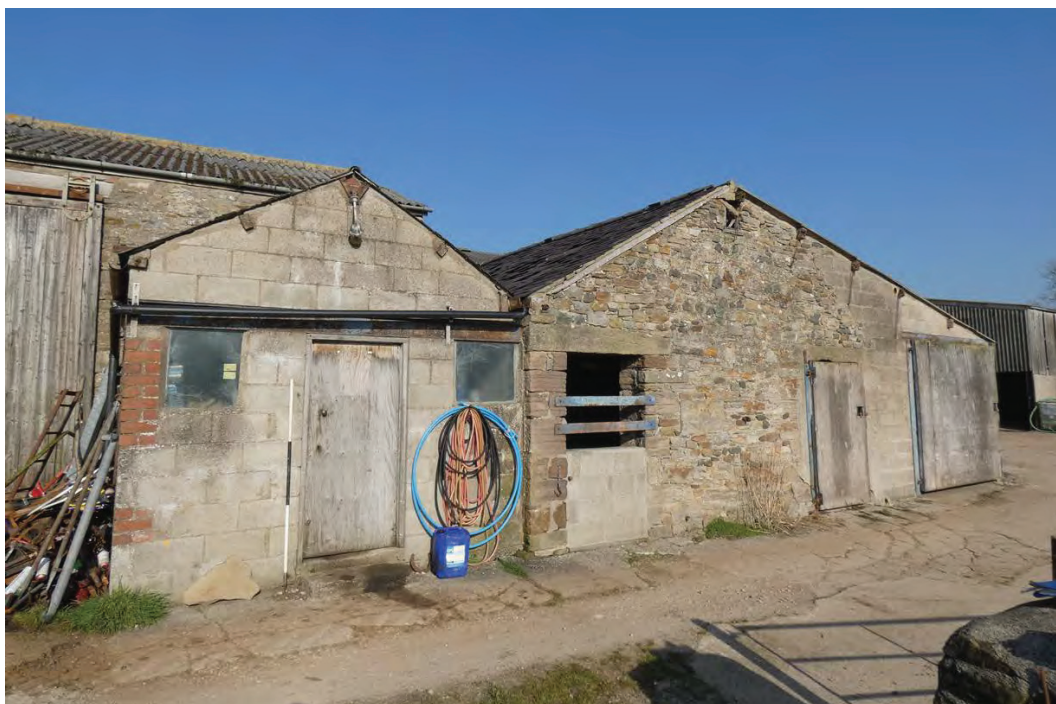
Plate 15: The north-east end of the south-east external elevation, viewed from the east
