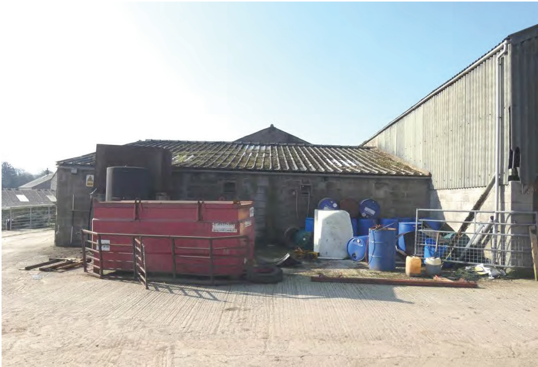
Plate 11: The south-east end of the north-east external elevation, viewed from the north-east
