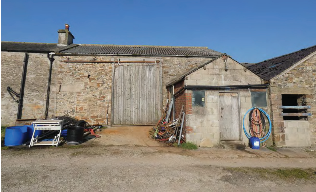
Plate 13 (left): The south-west end of the south-east external elevation, viewed from the south-east
