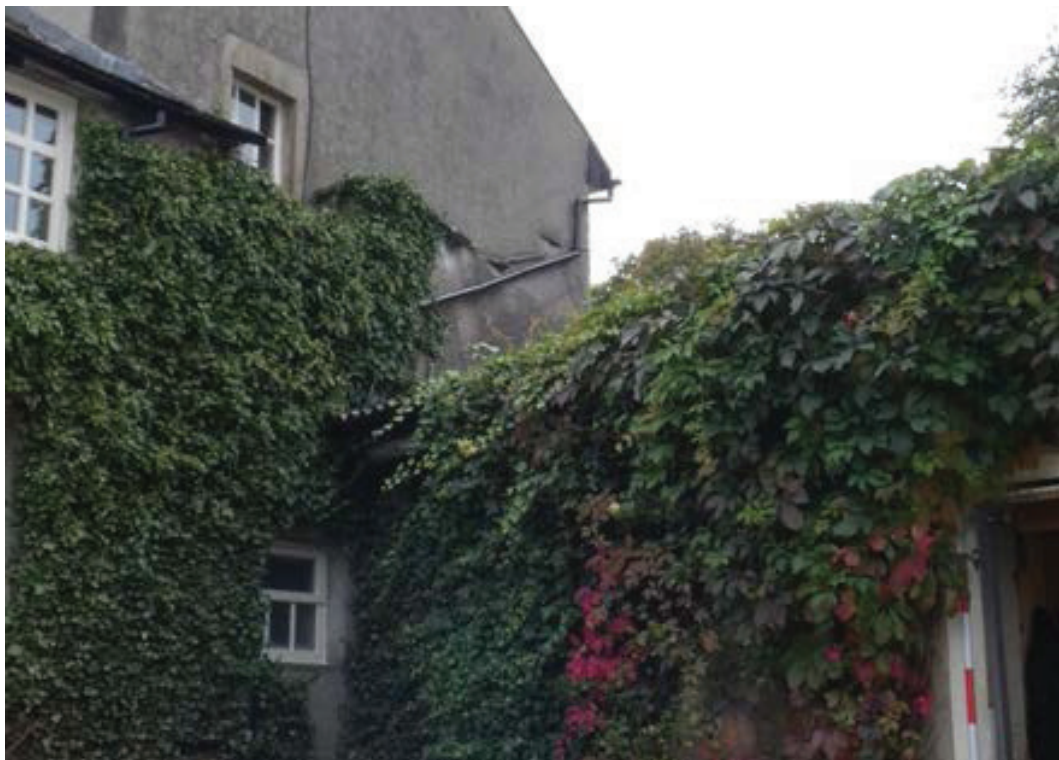
Plate 24: Details of the former roof line visible in the north-west external elevation of the adjoining building, viewed from the east
