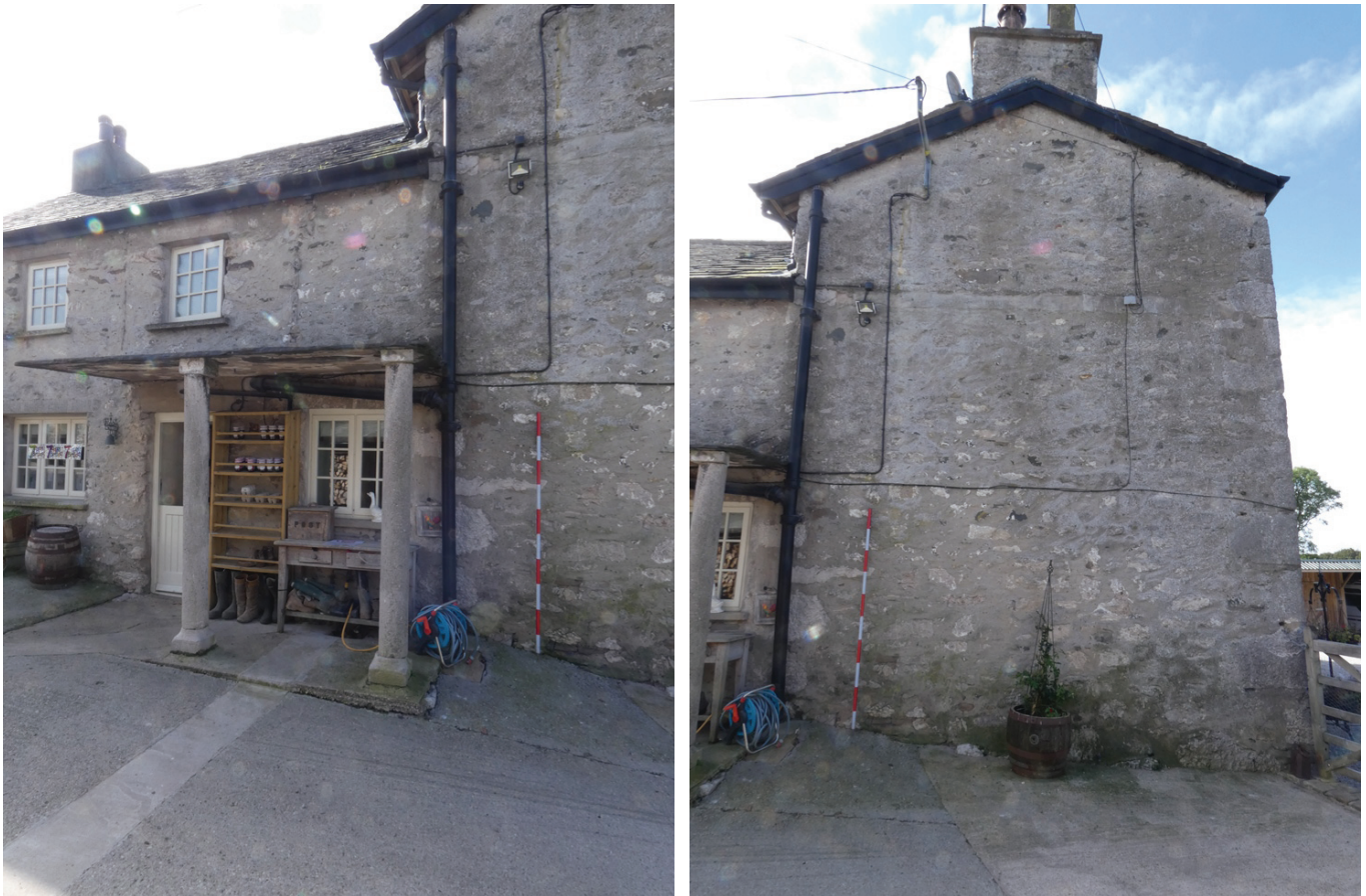
Plate 14 (left): The junction north-west end of the north-east external elevation, viewed from the north
