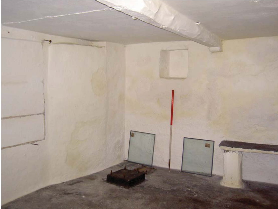
Plate 19: South-west corner of C1 showing bulge in wall, beam and blocked window
