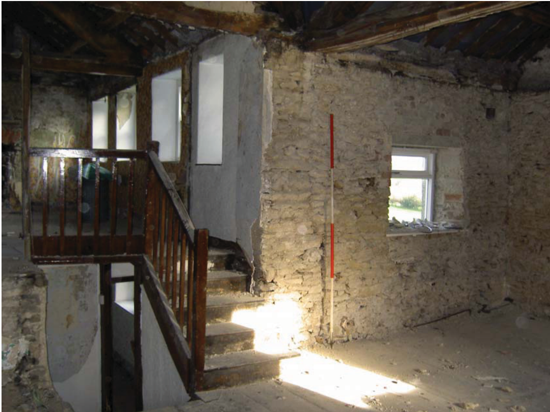
Plate 35: The east side of the north elevation of F1 showing the stairs and junction between the wall and the east side of the extension to the north
