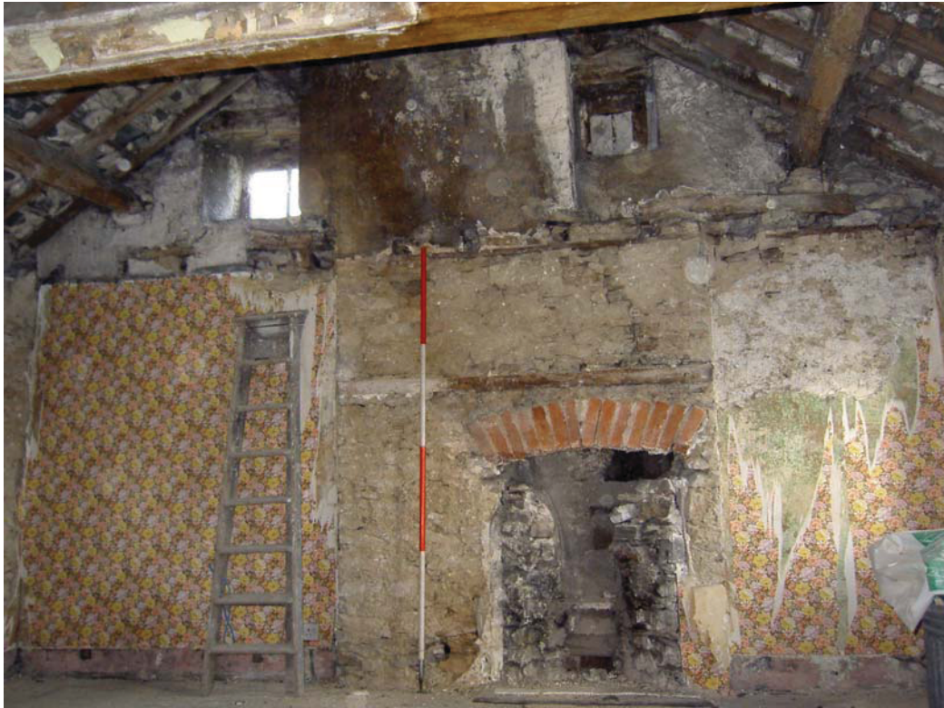
Plate 39: The fireplace and attic level windows in the north elevation of F2
