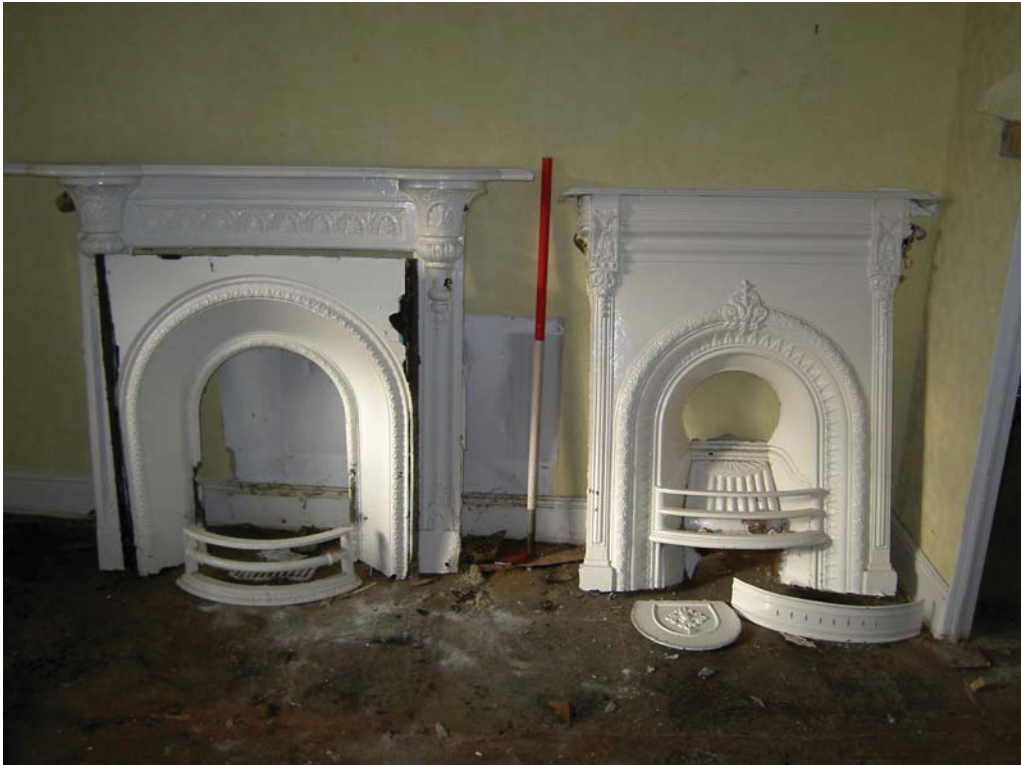
Plate 41: Loose cast iron fire surrounds in G2
