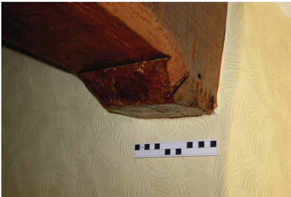
Plate 28: Detail of stop chamfer at south end of easternmost beam in G2
