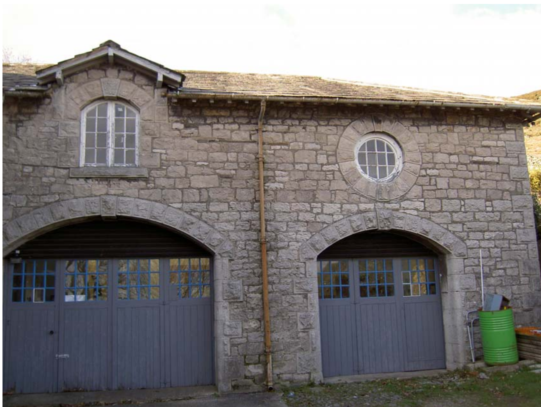
Plate 49: Front (south-east) elevation of the coach house showing the different styles of building above and below the doorways
