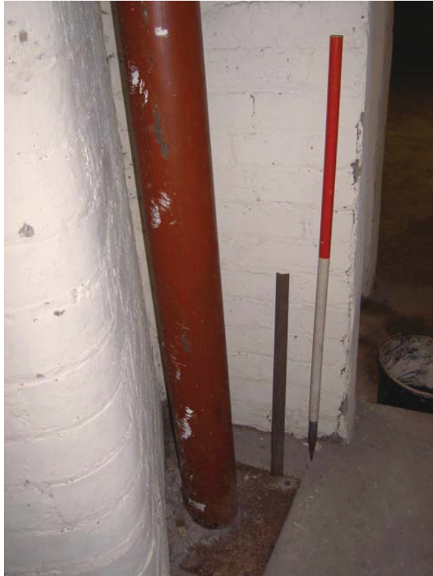
Plate 22: Base of the inserted post and raised concrete floor in the basement
