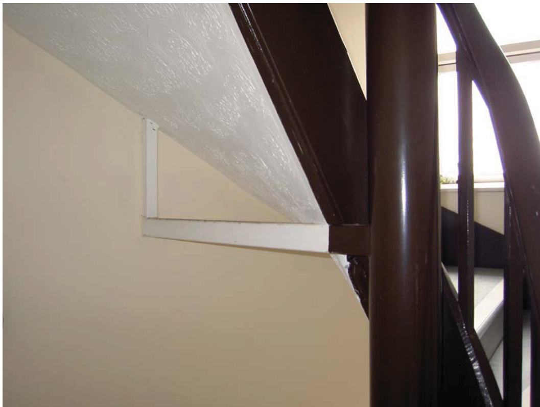
Plate 12: Horizontal bar and vertical strut extending from the inserted metal post on the second floor
