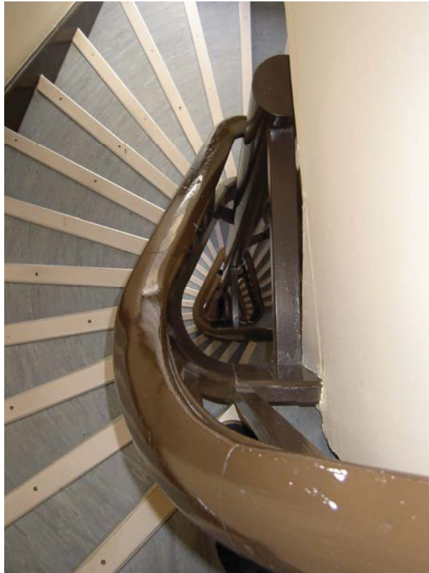
Plate 9: View down the stair well from the third floor showing the inserted post and horizontal bars
