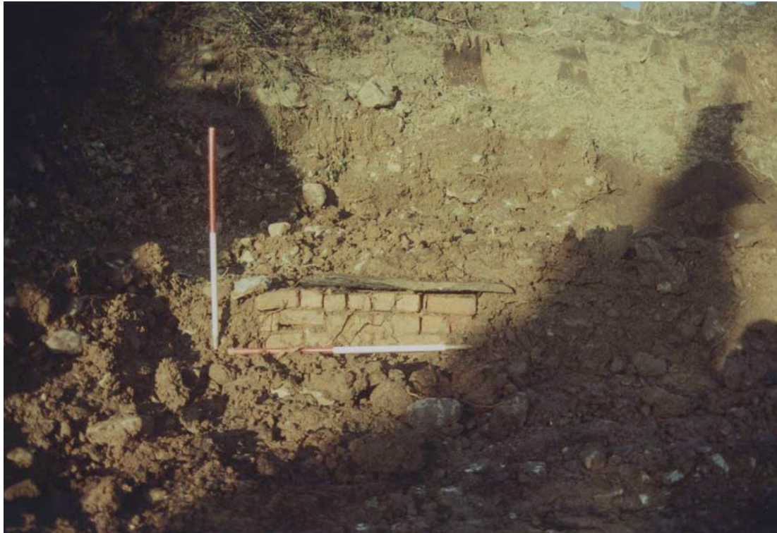
Plate 7: Brick drain junction capped with slate revealed behind the retaining wall during the watching brief
