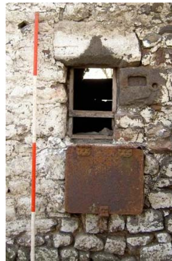
Plate 16: Re-used stone and iron container with lid forming a chute incorporated into a window in the west end of the north elevation of the barn
