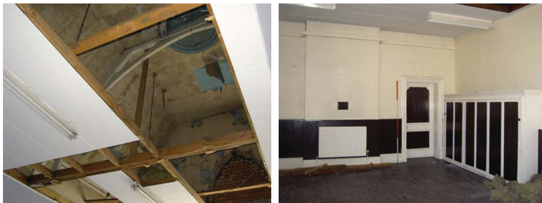
Plate 35: (left) Elaborate roof structure and blocked Gothic arch visible above suspended ceiling in Room 3
