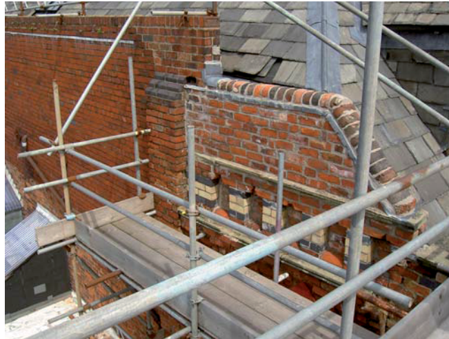
Plate 25: Detail of the south-east corner of the south-west elevation, showing decorative brickwork and repairs
