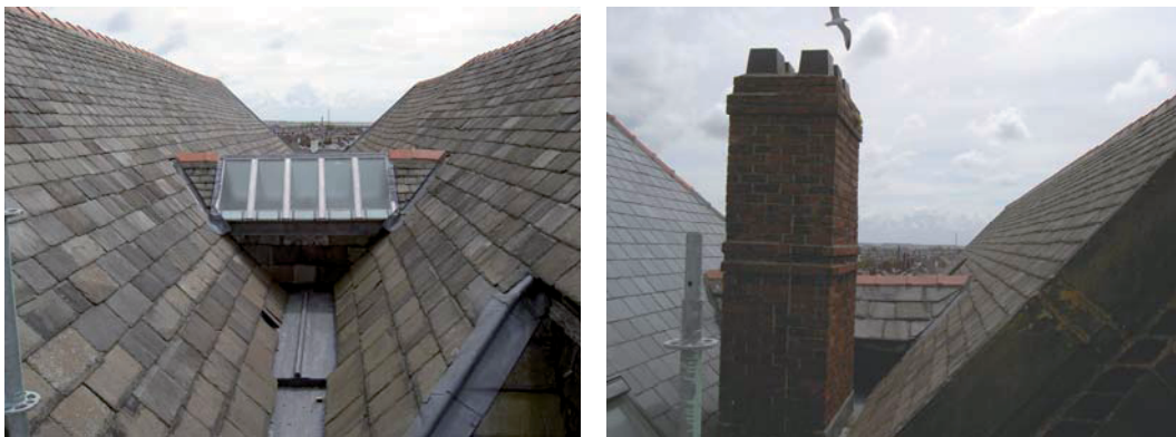
Plate 30: (left) Roof of connecting corridor between attic floor Rooms 1a and 2a, viewed from the north-west
