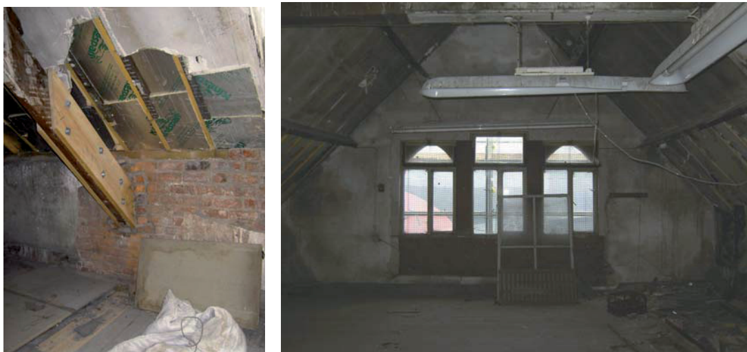
Plate 88: (left) Attic Room 2a, detail of repair to south-west end of south-east truss
