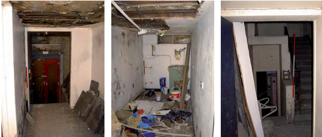
Plate 38: (left) Area S1, centre of the south-east elevation, showing door to High Street (left)
