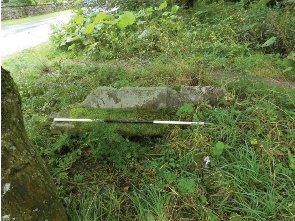
Plate 12: Possible sluice gate at the south-west end of the structure, viewed from the south-west
