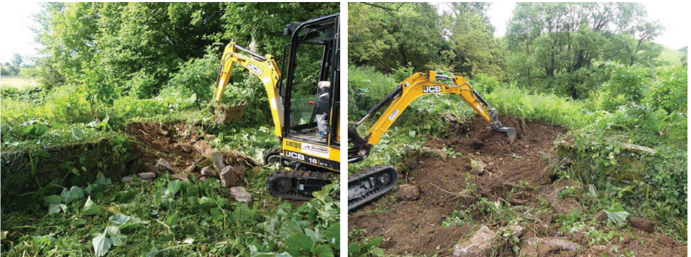
Plate 14 (left): Working shot showing the excavator cutting through the former mill leat, viewed from the north
