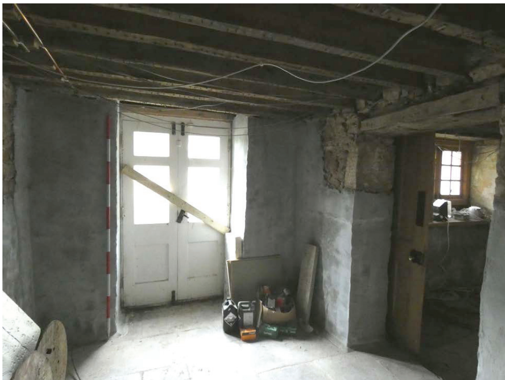
Plate 45: Doorways in the south and west elevations of lower ground floor Room 5, viewed from the north-east
