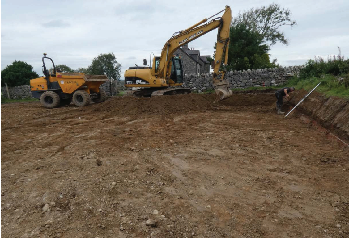
Plate 14: Excavating the electricity cable by hand to the north end of the area
