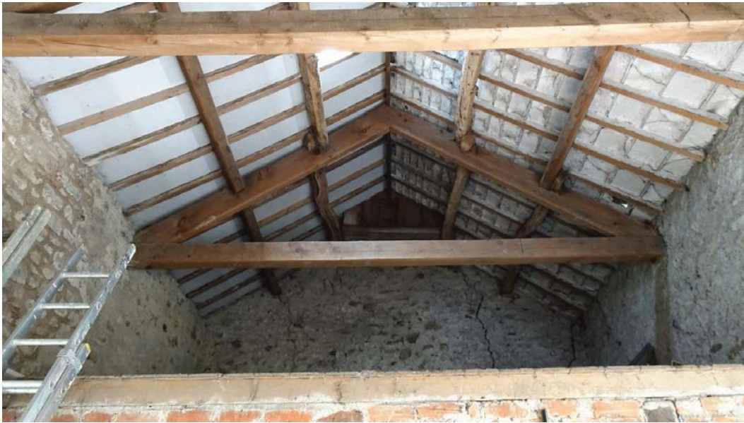
Plate 9: Tie beam truss at the north end of the main section of the building, viewed from the south
