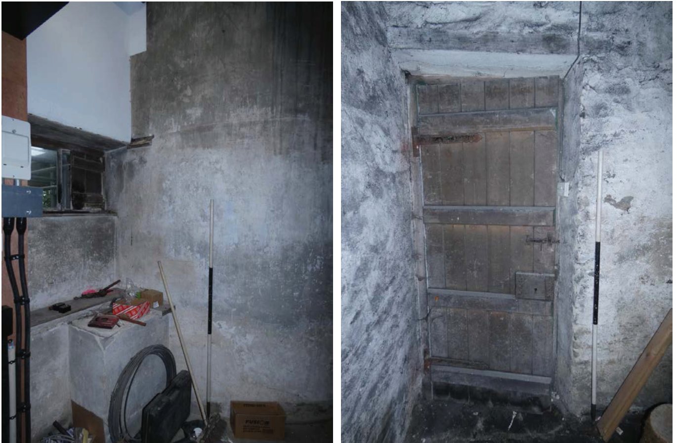
Plate 62 (left): The curved section in the west elevation of Room G10, viewed from the north-east
