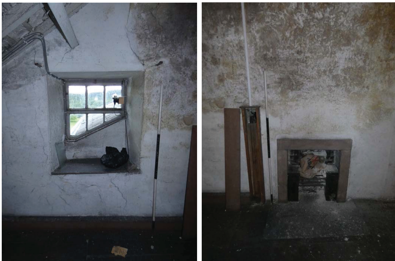
Plate 116 (left): The window in the west elevation of Room S5, viewed from the east
