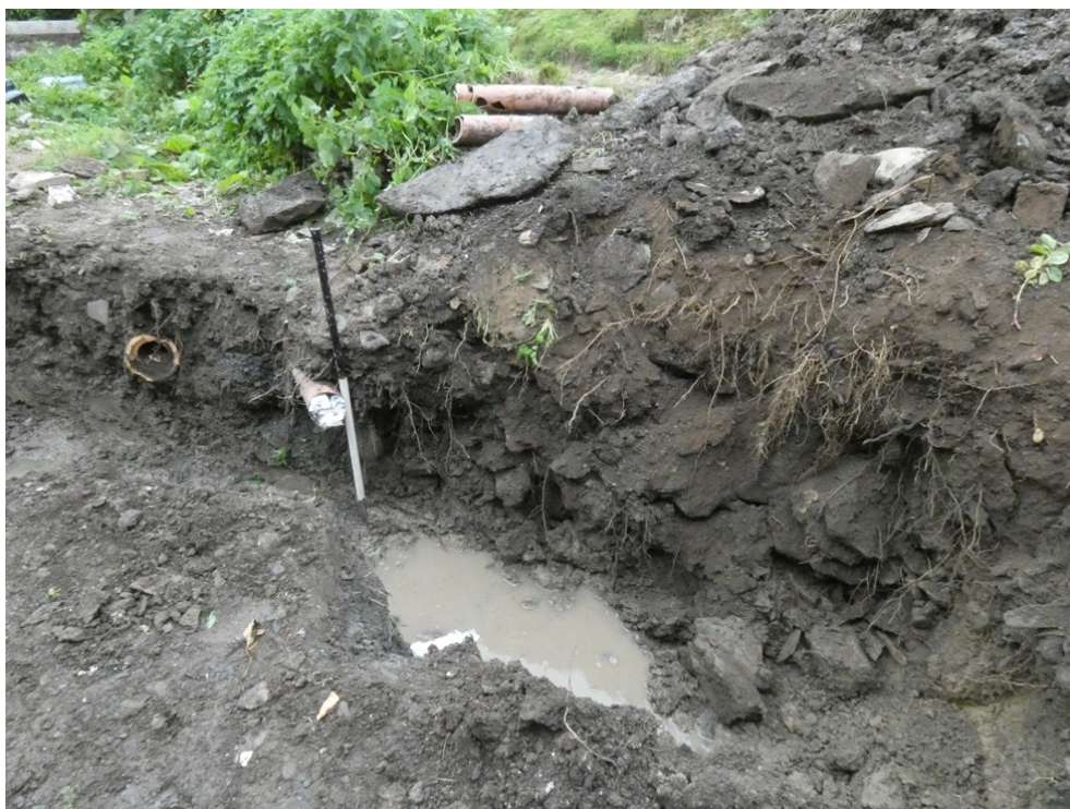
Plate 9: The deposit of large stones, part of deposit 103, exposed in the western foundation trench, viewed from the north-east
