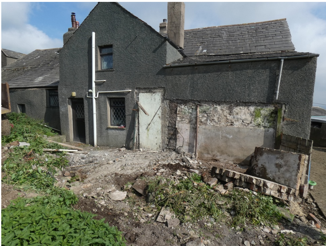
Plate 7: The site following the demolition of the outshuts but prior to any groundworks, viewed from the south-west
