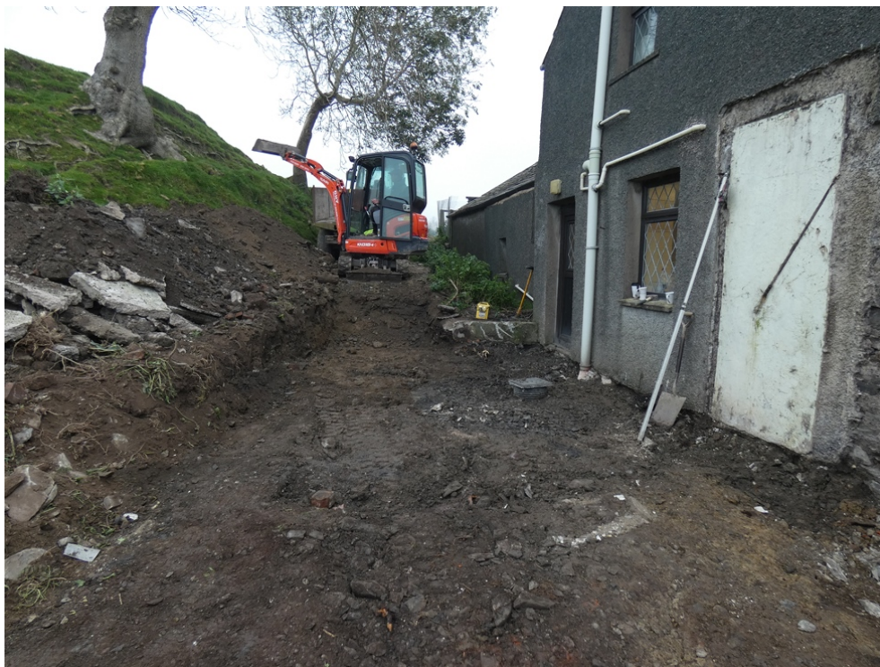
Plate 8: The site following initial levelling, showing the extent of deposit 103, viewed from the south
