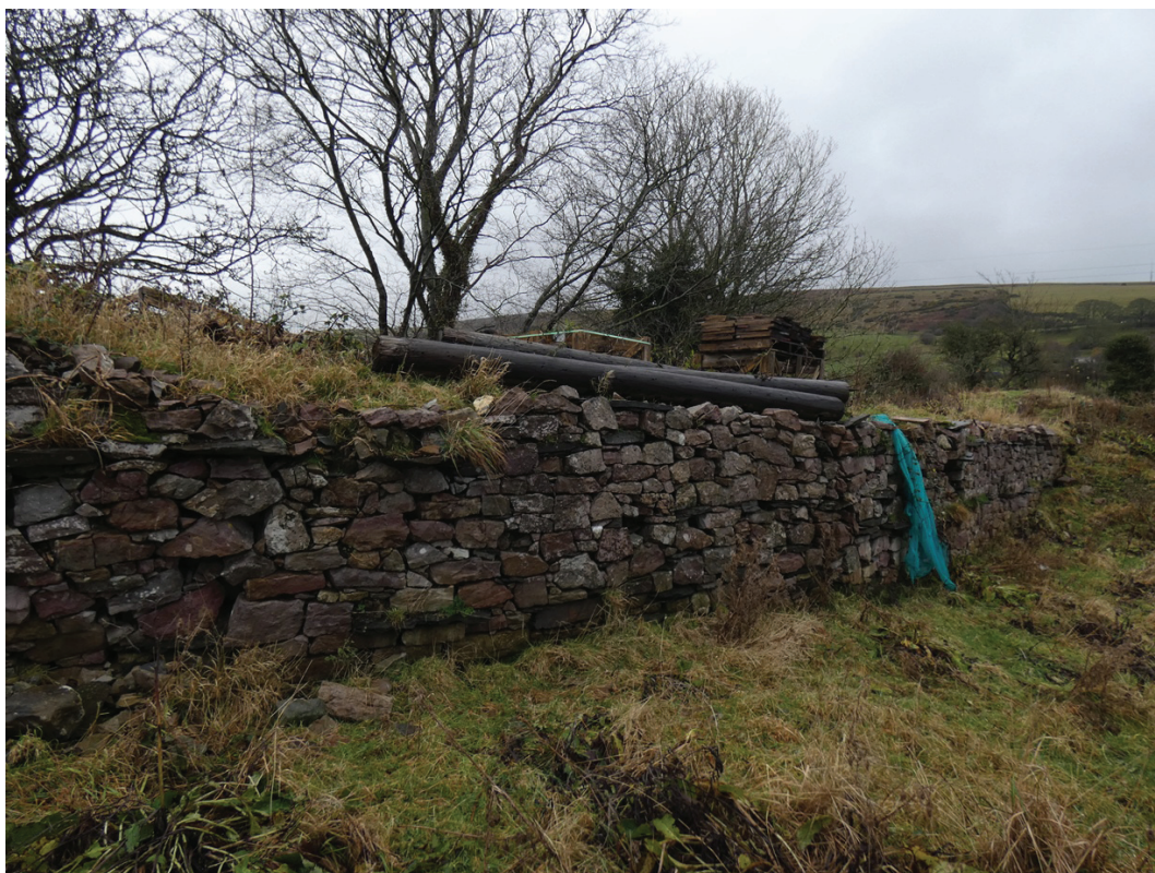
Plate 11: Retaining wall to the east of the water wheel, viewed from the south-west
