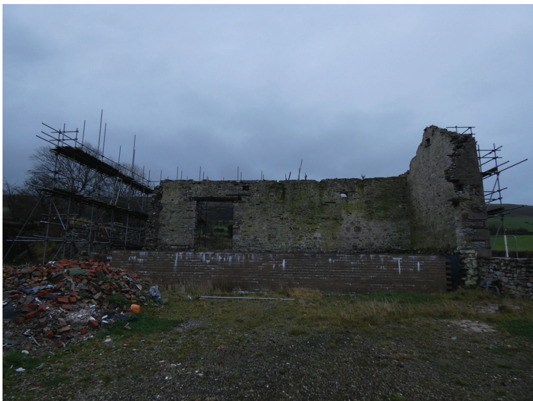
Plate 6: The main barn viewed from the west, showing the missing west wall and new foundations
