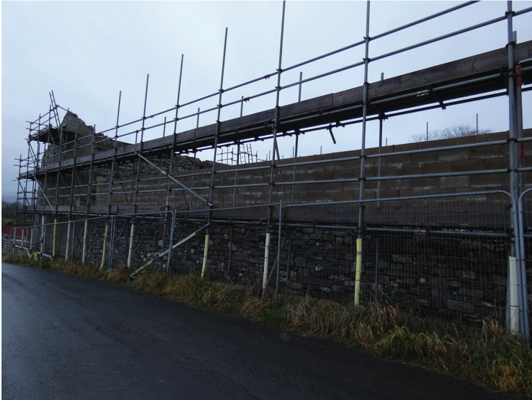
Plate 8: The rebuilt south wall of the eastern outshut, viewed from the south-east
