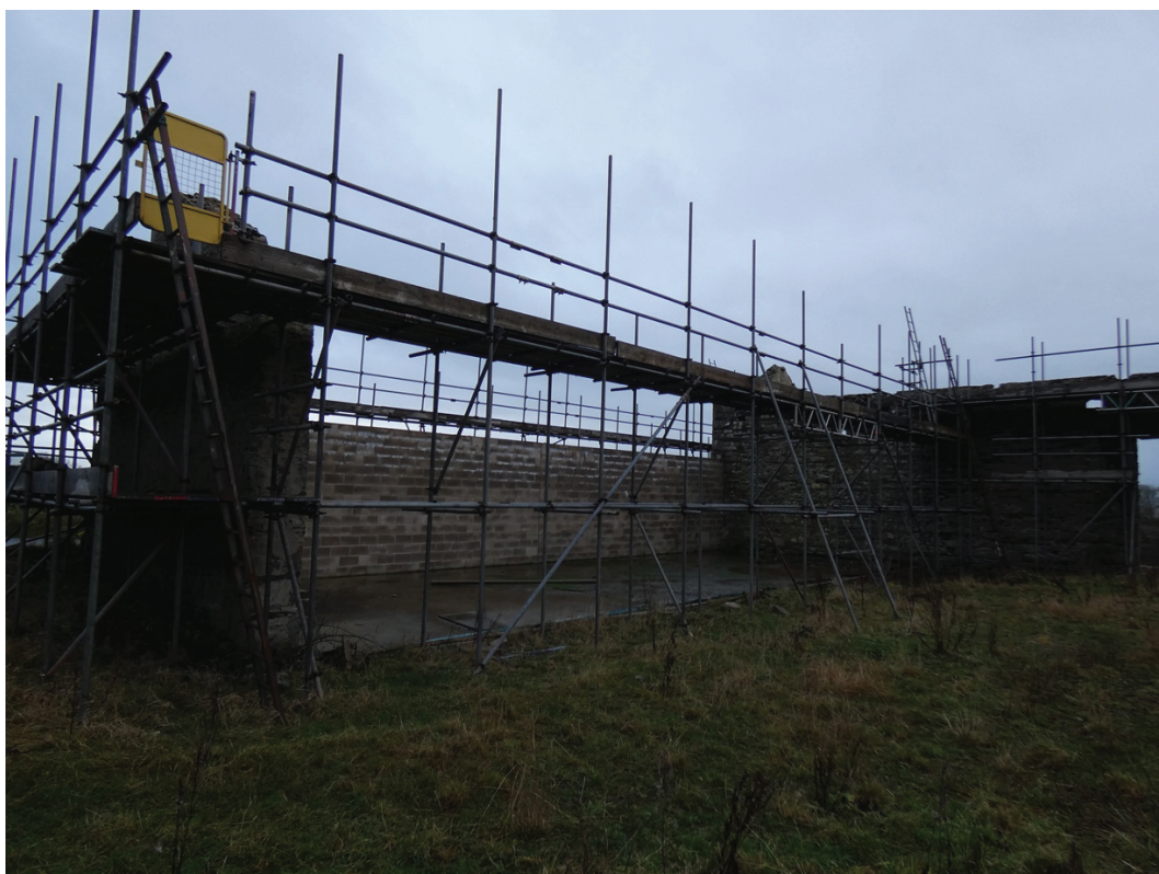
Plate 7: The outshut to the east, viewed from the north-east, showing the new wall and concrete floor
