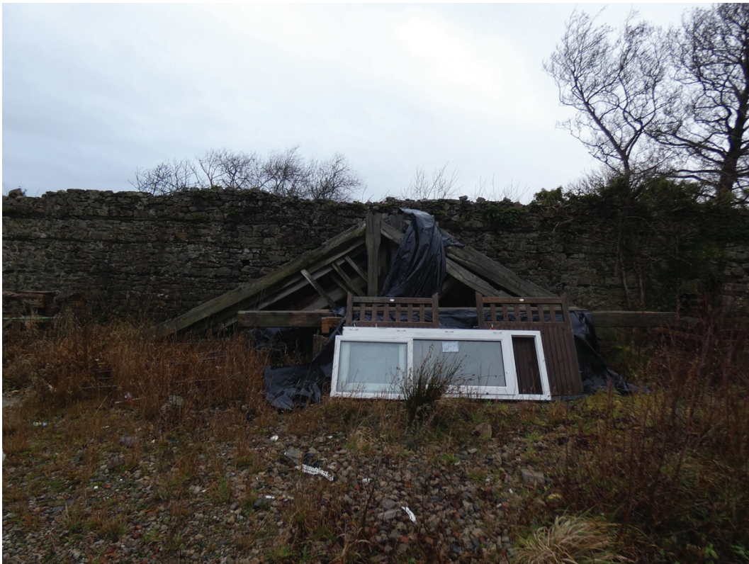
Plate 9: Roof trusses lose on site against the west boundary wall, viewed from the east
