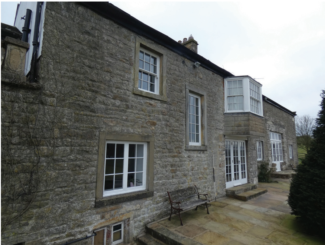
Plate 24: General view of the central part of the west external elevation, viewed from the north-west
