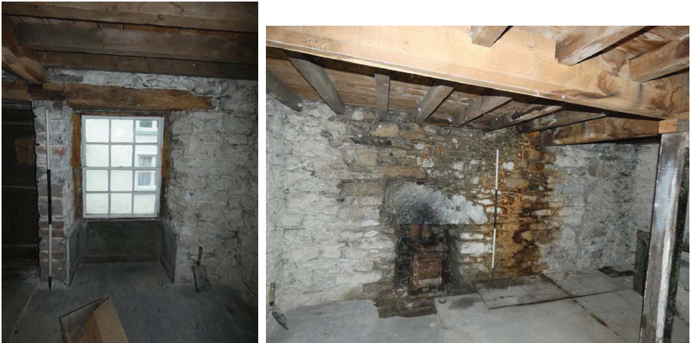
Plate 41 (left): Window on the north-east side of the north-west elevation, Room F1, viewed from the south-east
