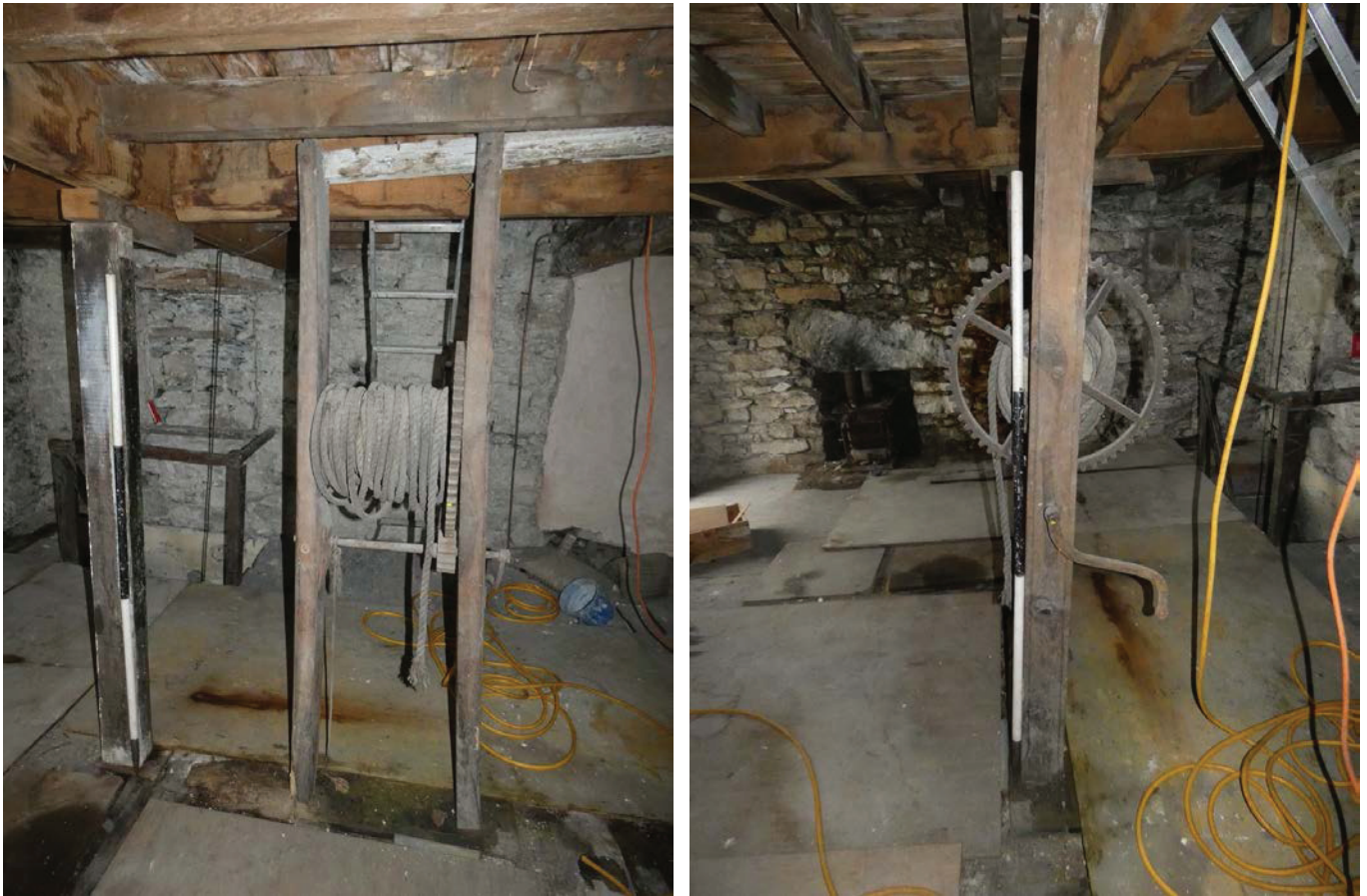
Plate 35 (left): Hoist winch in Room F1, viewed from the north-west
