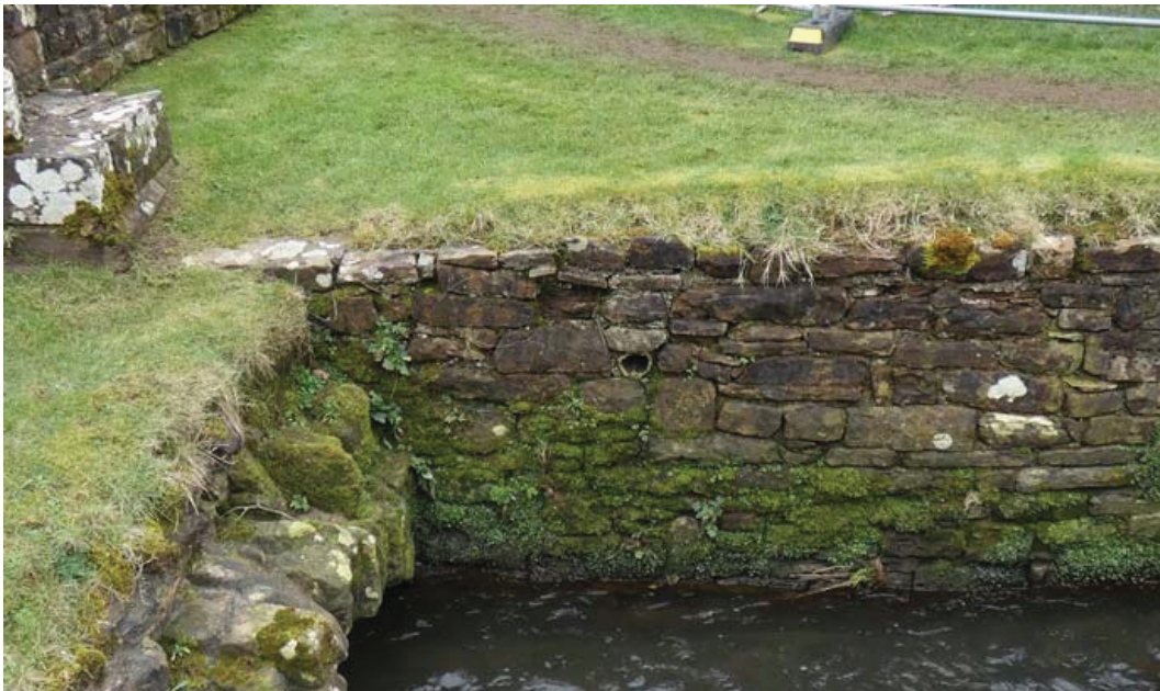
Plate 7: Pipe visible in section in the culvert wall, viewed from the north-east
