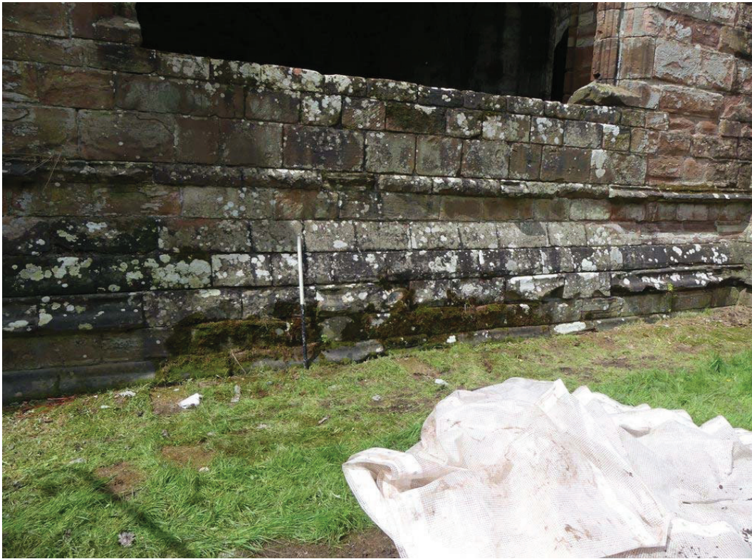
Plate 16: The east end of the infirmary chapel, showing the removed mouldings, viewed from the south-east
