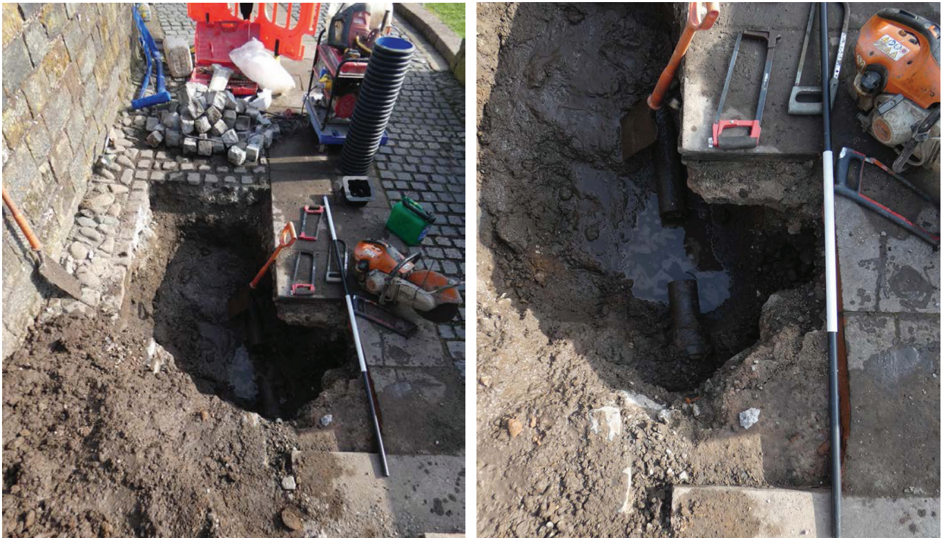
Plate 7 (left): The damaged pipe exposed and cut through
