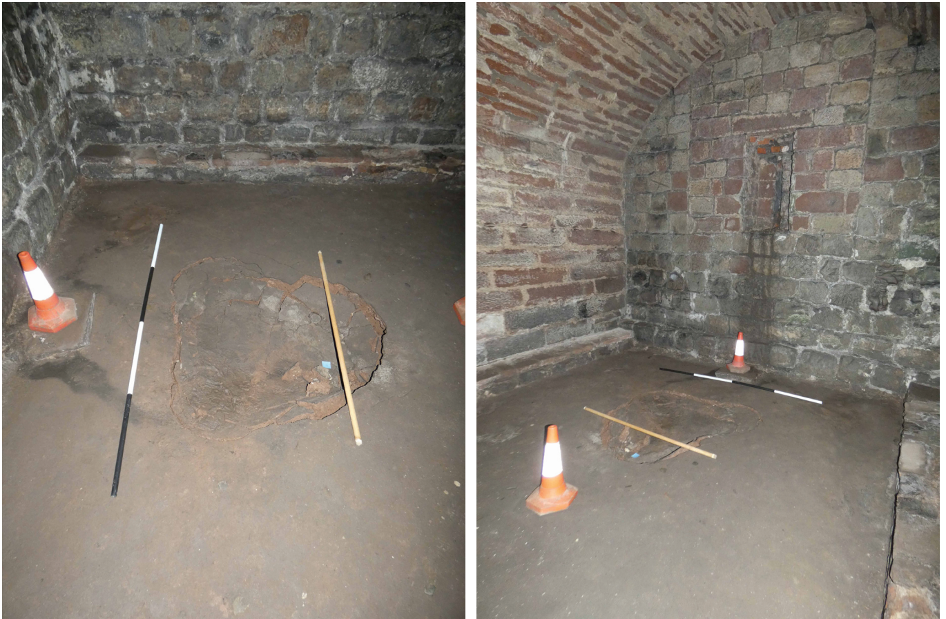
Plate 4: Area of collapse in the dungeon / storeroom, viewed from the north-east
