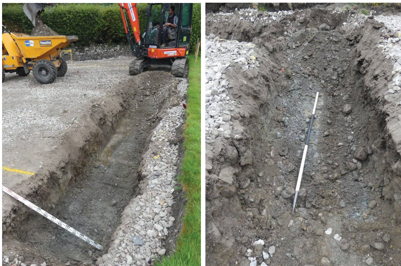
Plate 20 (left): Grey natural (1008) exposed at the south-east corner of the garage footings
