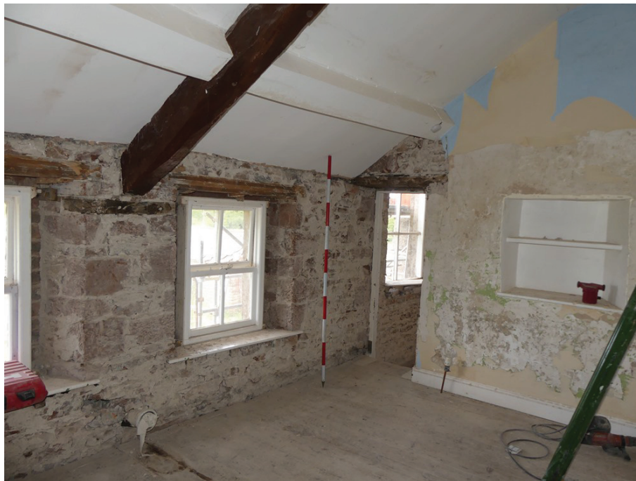
Plate 66: The south-west and north-west elevations in Room F2, viewed from the east
