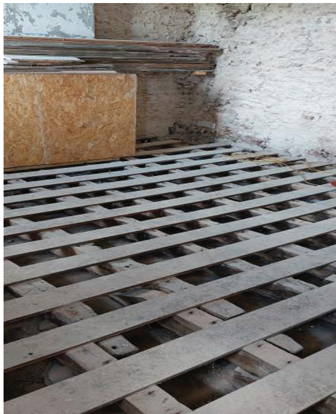
Figure 2c/d: View of rooms G5 (top) and G7 (bottom) to help locate sampled timbers (see Fig 3c & Table 1)
