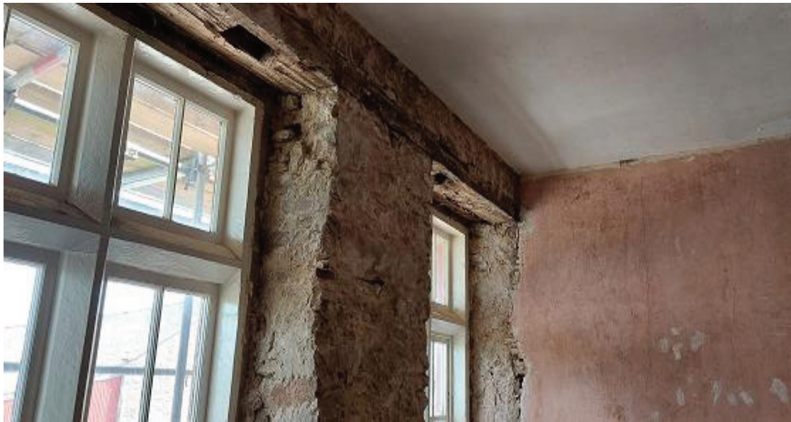
Figure 2a/b: View of rooms G1 (top) and F4 (bottom) to help locate sampled timbers (see Figs 3a/b & Table 1)
