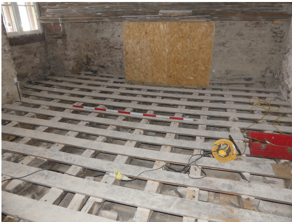
Plate 48: General view of the floor of Room G7, viewed from the south
