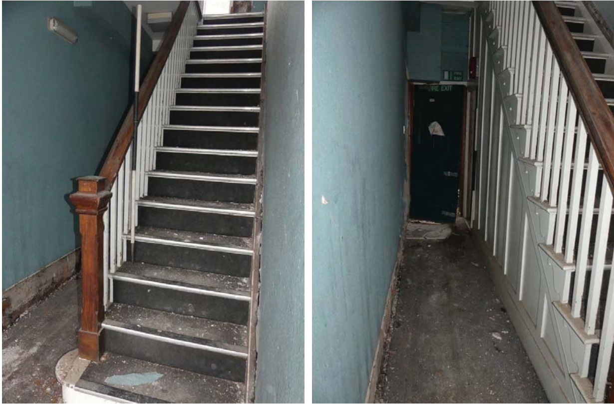
Plate 79 (left): The stairs in Room G14 of the police station, viewed from the south-east
