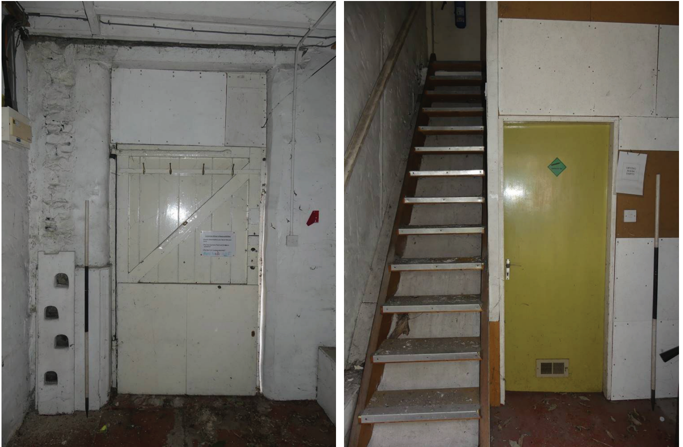
Plate 126 (left): The north-west elevation of Room G11 of the courthouse, viewed from the south-east
