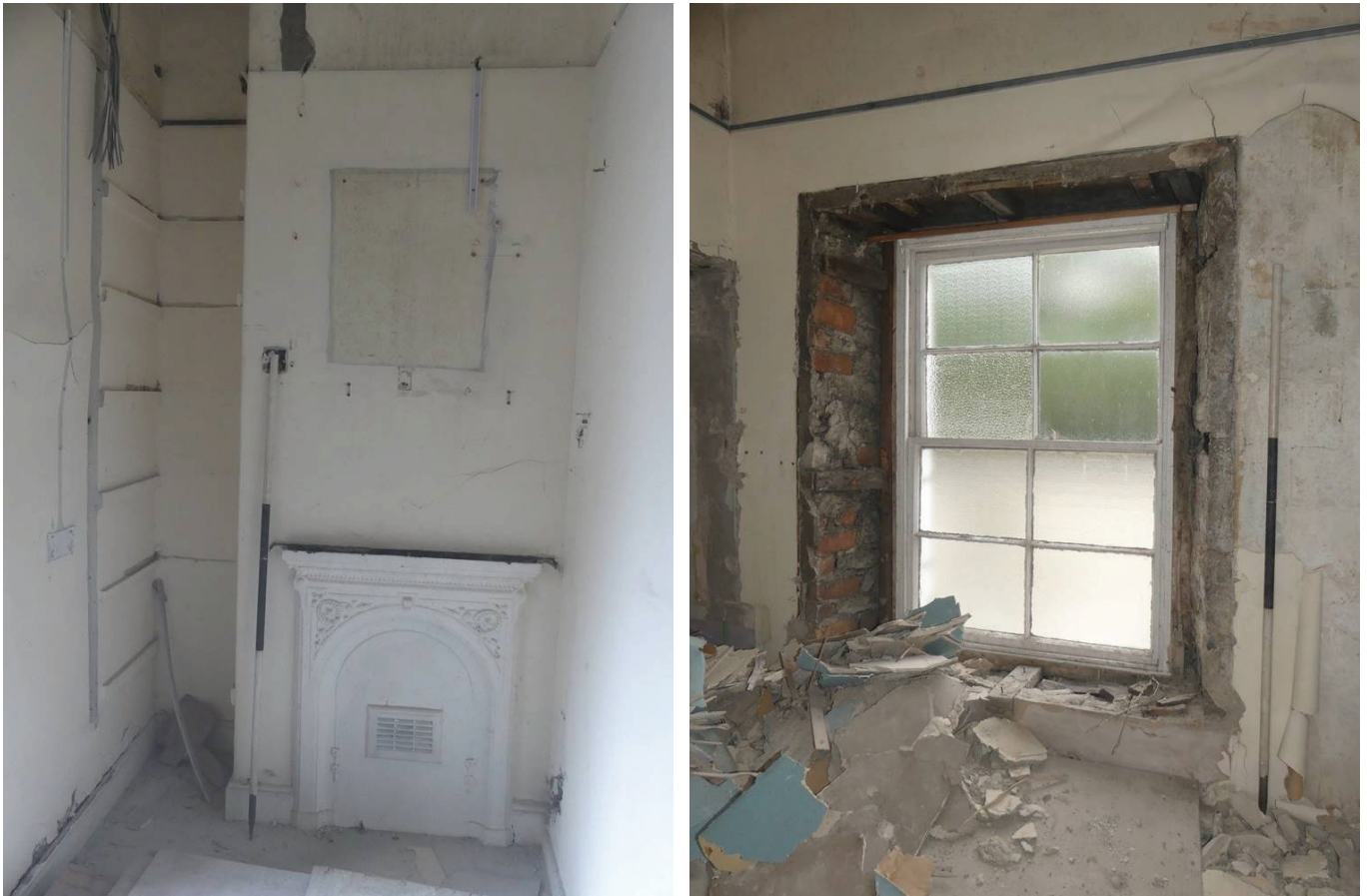
Plate 99 (left): The south-west elevation in Room F6 of the police station, viewed from the north-east
