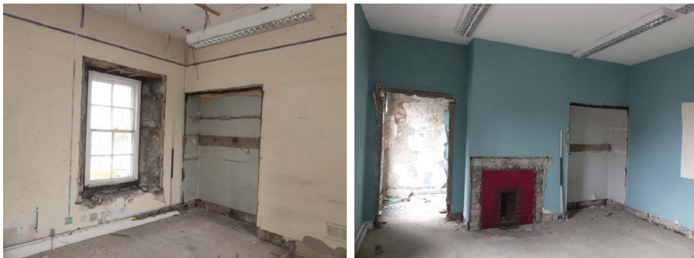
Plate 101 (left): General view of Room F8 of the police station, from the south
