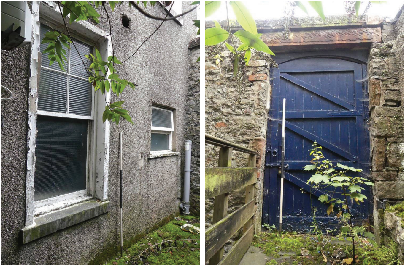
Plate 23 (left): Ground floor windows on the south-west side of the north-west external elevation of the police station, viewed from the north
