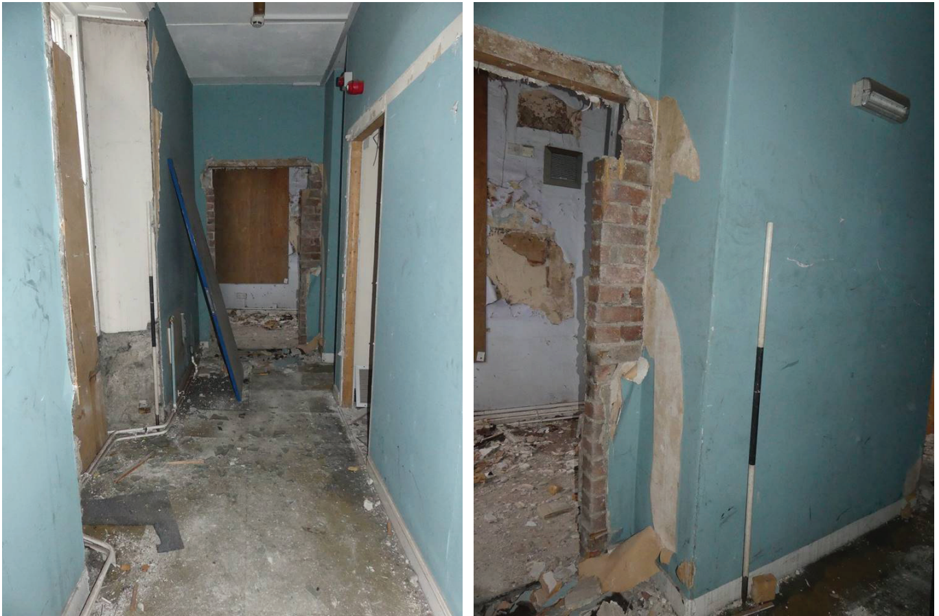
Plate 83 (left): General view of Room G15 of the police station, from the north-east
