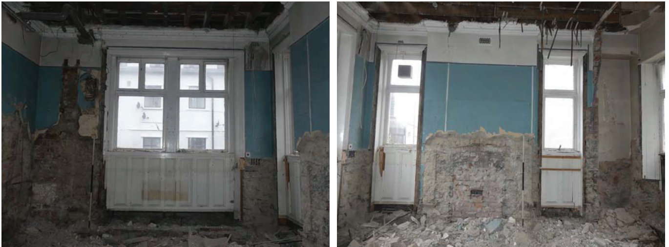
Plate 60 (left): The north-east elevation of Room G1 of the police station, viewed from the south-west
