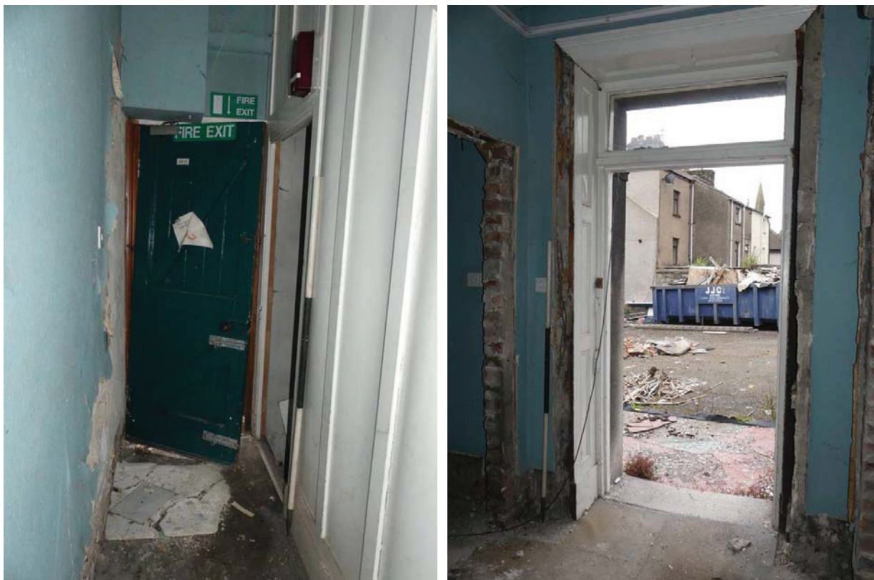
Plate 81 (left): Doorway to the north-west in Room G14 of the police station, viewed from the south-east
