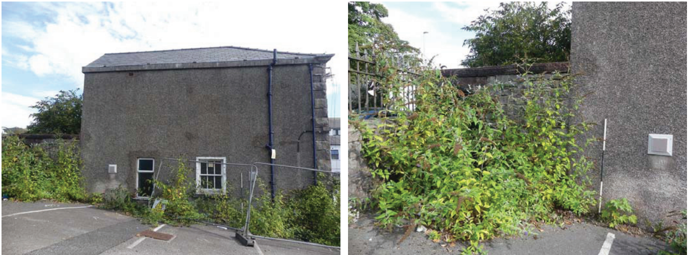
Plate 29 (left): The south-west external elevation of the police station, viewed from the south-west
