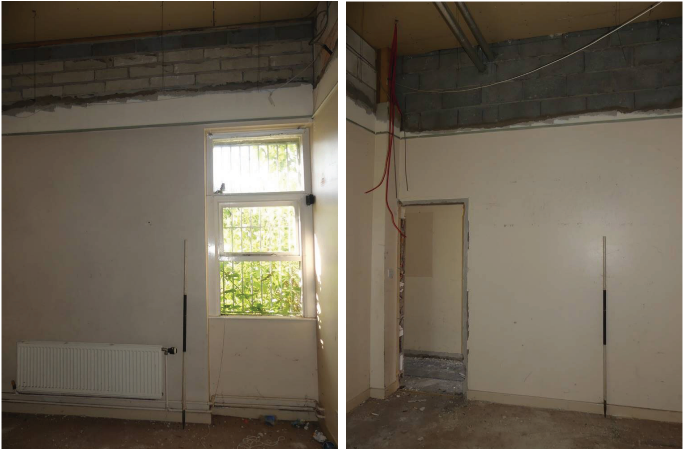
Plate 113 (left): The south-west elevation in Room G4 in the courthouse, viewed from the north-east
