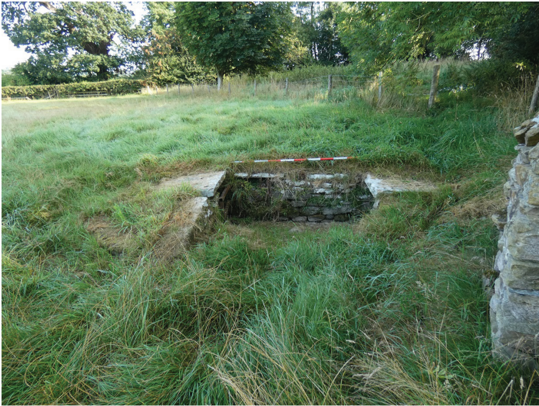
Plate 23: Stone-lined channel to the east of the proposed riding surface, viewed from the south
