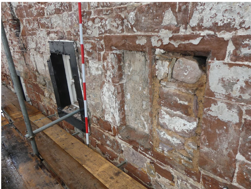
Plate 27: The blocked mullion window at first floor level in the south-east elevation, viewed from the south
