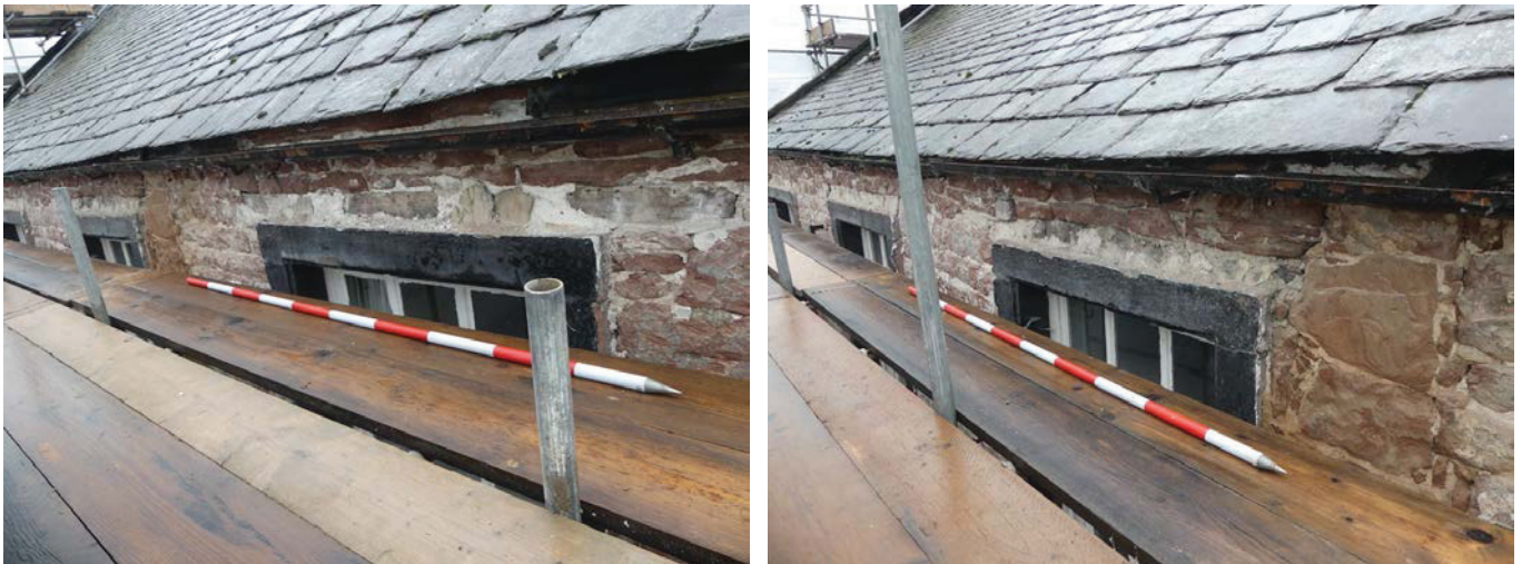
Plate 5 (left): Window tops showing clad lintels at the top of the north-east elevation, viewed from the north Plate 6 (right): Window tops showing clad lintels at the top of the north-east elevation, viewed from the north
