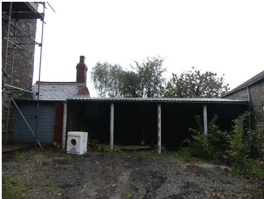
Plate 16: The north-east section of the north-west external elevation, viewed from the north-west
