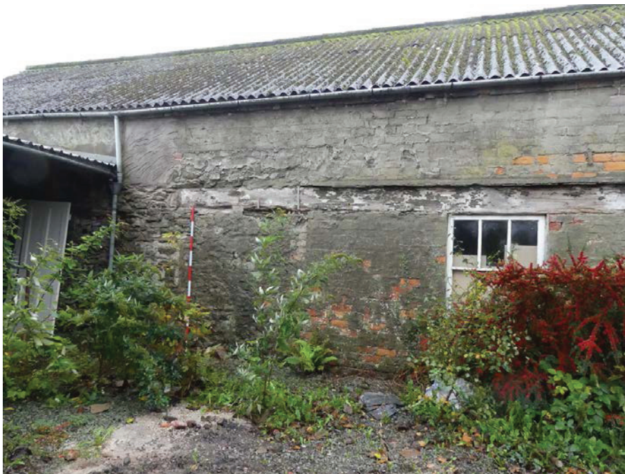
Plate 19: The blocked doorway in the north-east external elevation, viewed from the north-east
