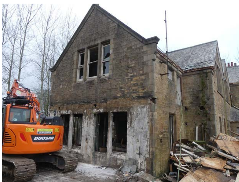
Plate 26: The south external elevation following the demolition of the later extension, viewed from the south-east
