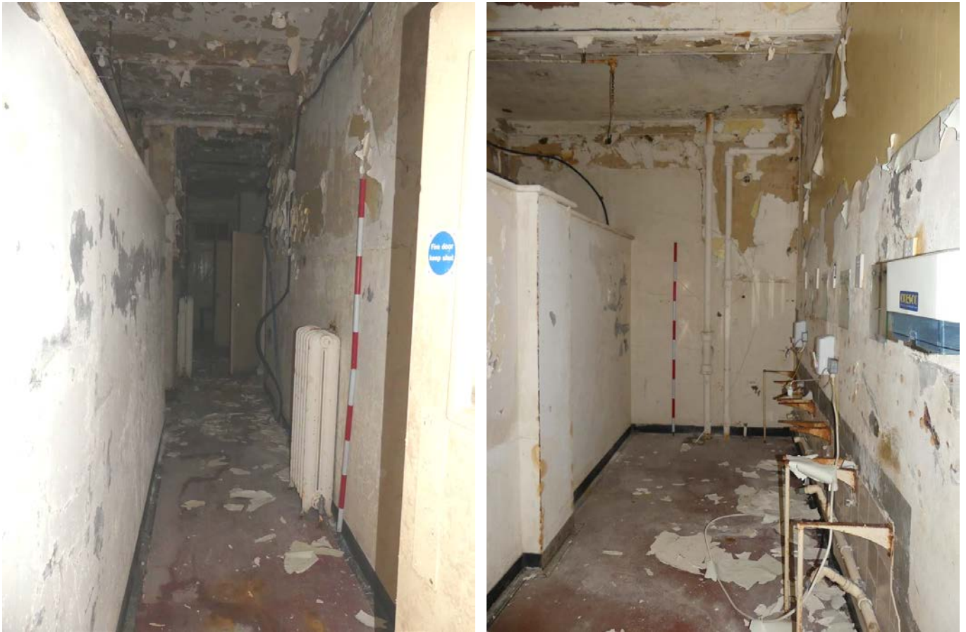
Plate 60 (left): The corridor along the east side of Room G9, viewed from the south
