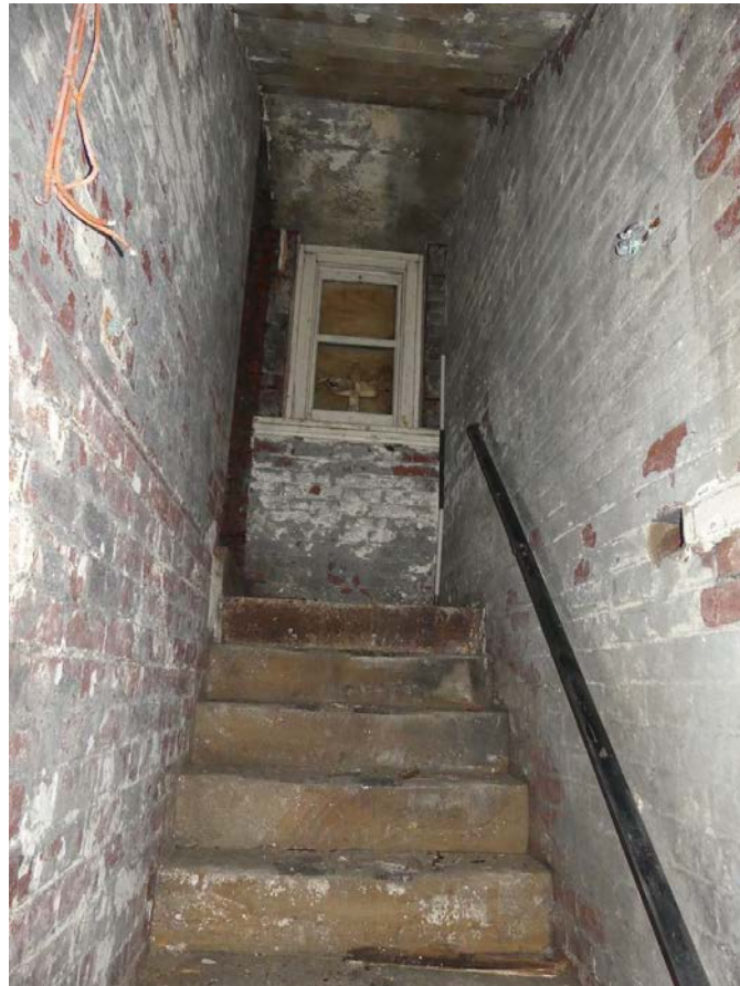
Plate 33: Stairs from the west side of the basement, viewed from the south
