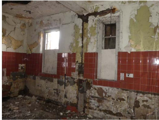
Plate 57: General view of the west side of Room G7, from the north-east
