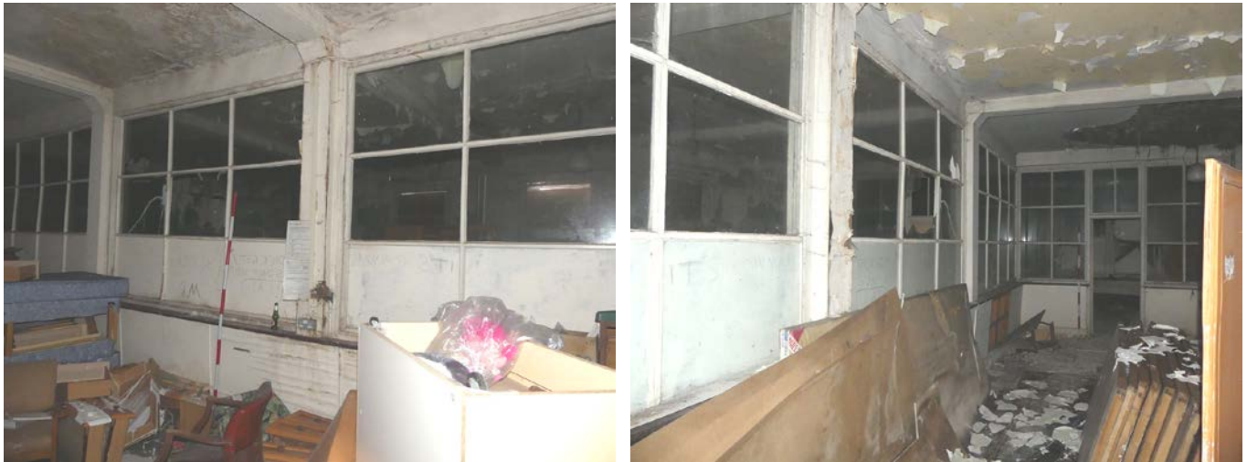
Plate 47 (left): The dividing stud partition wall between Rooms G3 and G4, viewed from the north-east in Room G3
