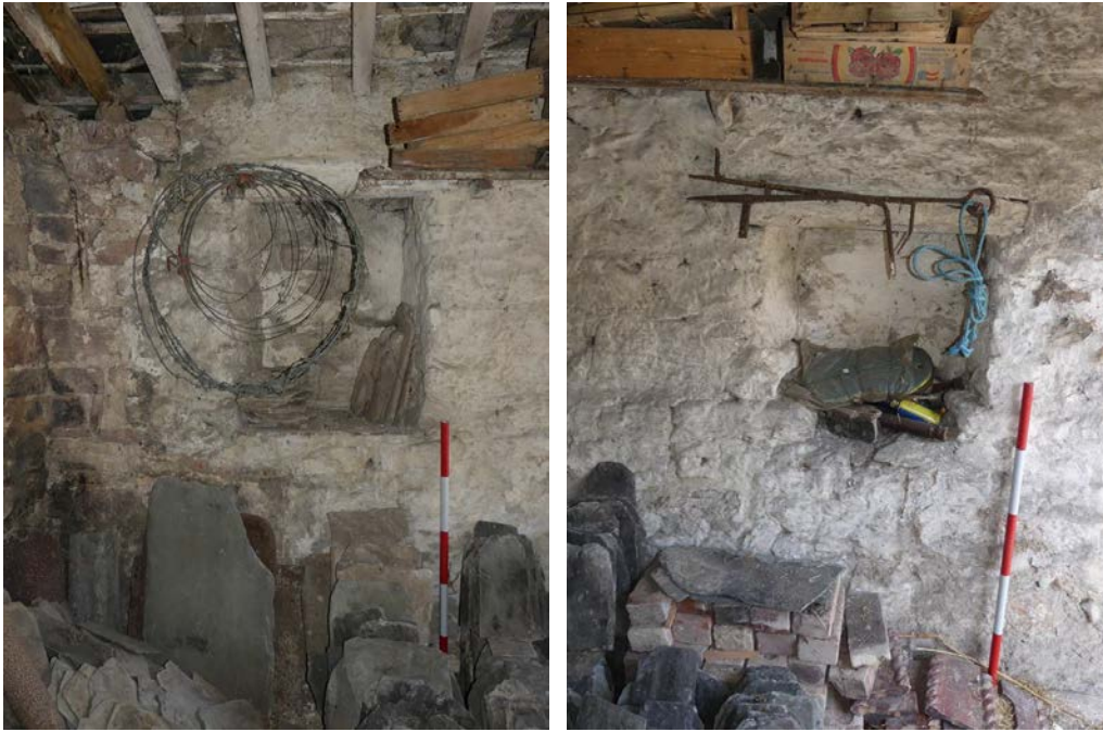
Plate 46 (left): Alcove to the west side of the north elevation in Room G4
