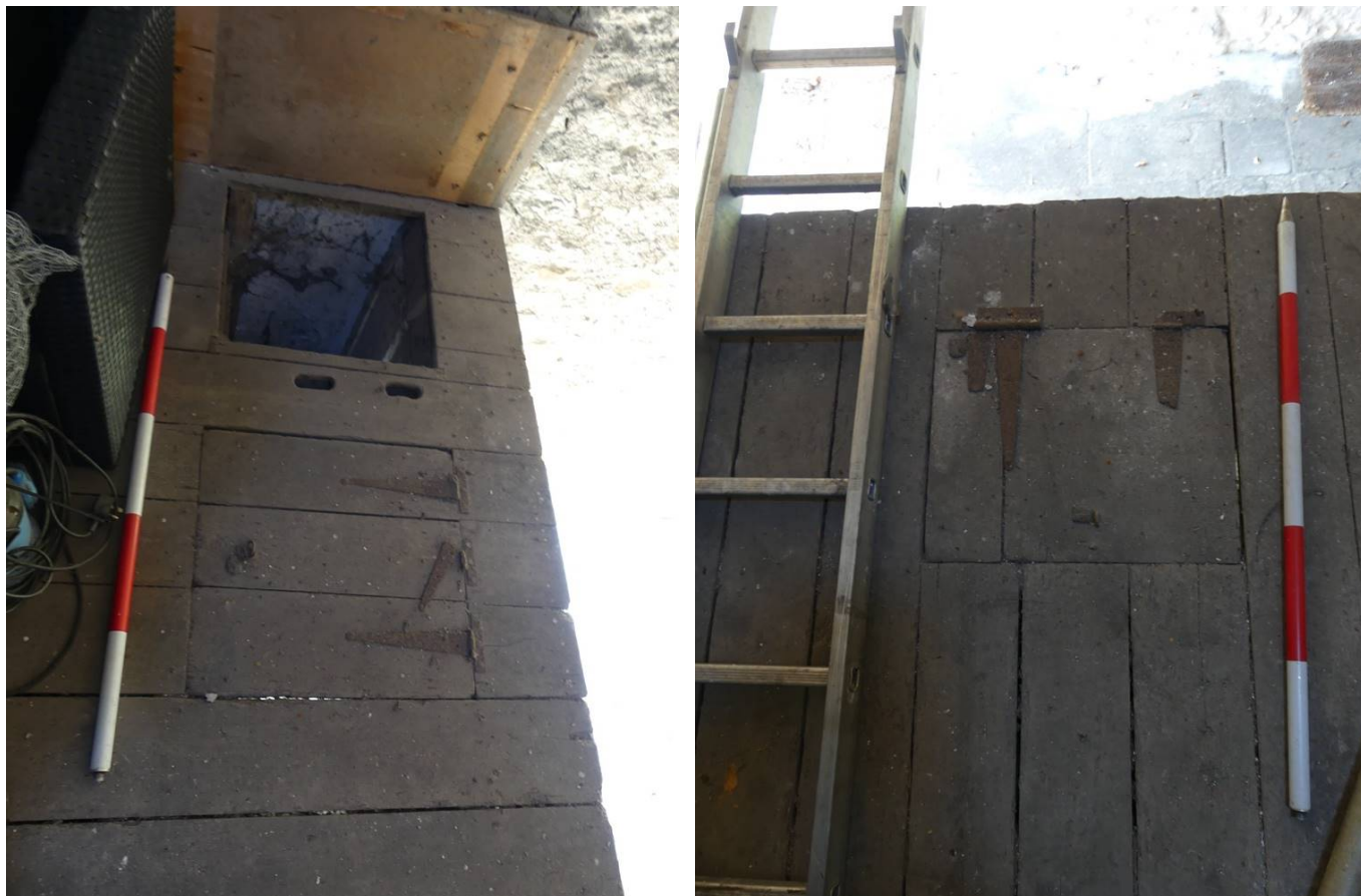
Plate 53 (left): Two hatches to the east side of the floor in Room G1
