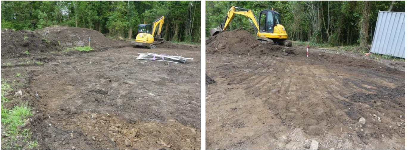
Plate 6 (left): Disturbed area on the west side of the site, viewed from the south-west
