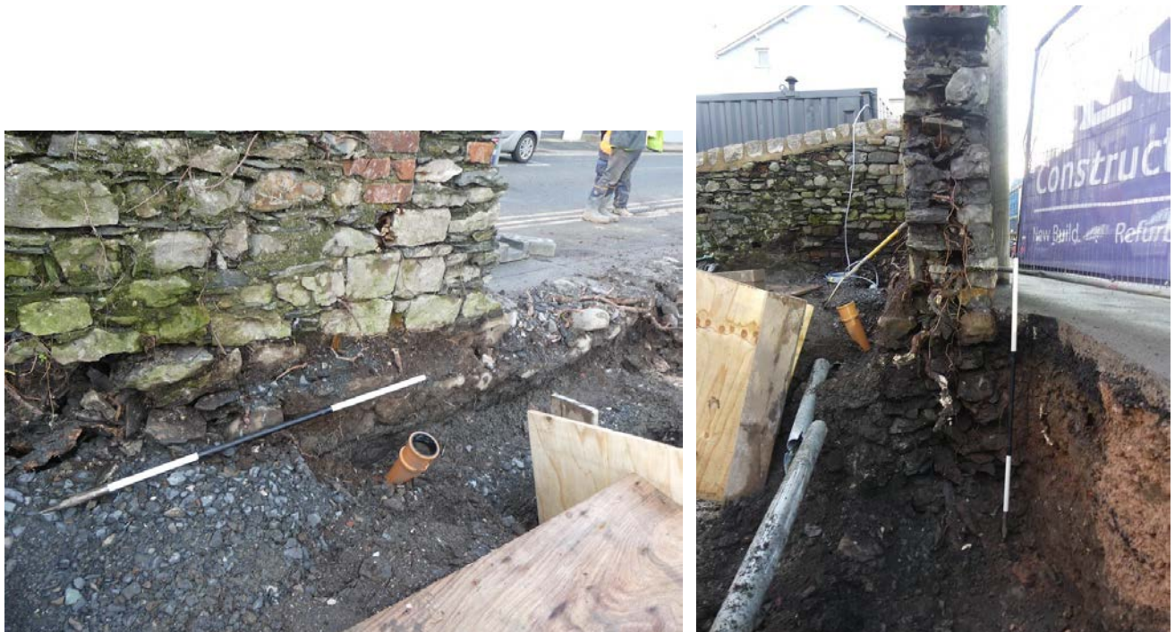
Plate 23 (left): North-west boundary wall and earlier foundation (2012) to the south-east, viewed from the south
