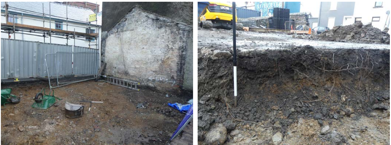
Plate 9 (left): Deposits revealed following the demolition of buildings to the east of the former Union Inn, viewed from the west
