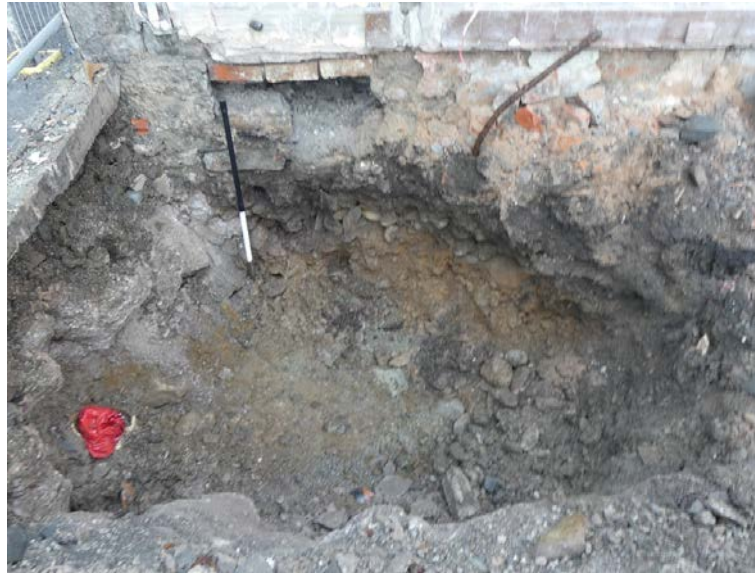
Plate 11: Deposits revealed following the demolition of the outshuts to the south-west of the former Union Inn, viewed from the south-east
