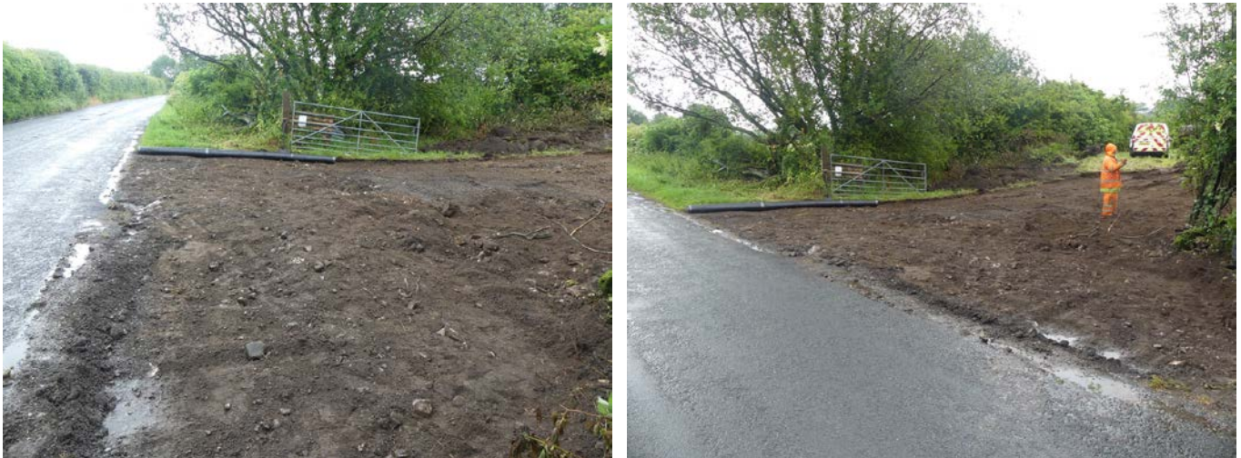
Plate 17 (left): Stripping at the north end of the haul road to create the new entrance, viewed from the south-west
