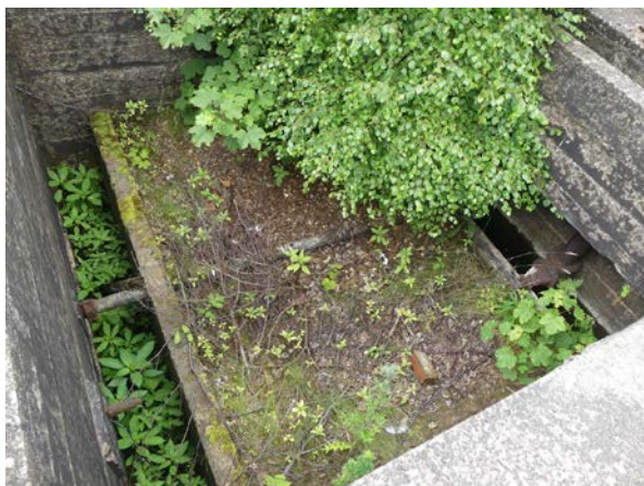
Plate 53: Base of the concrete tank to the west of the central tank, Area B
