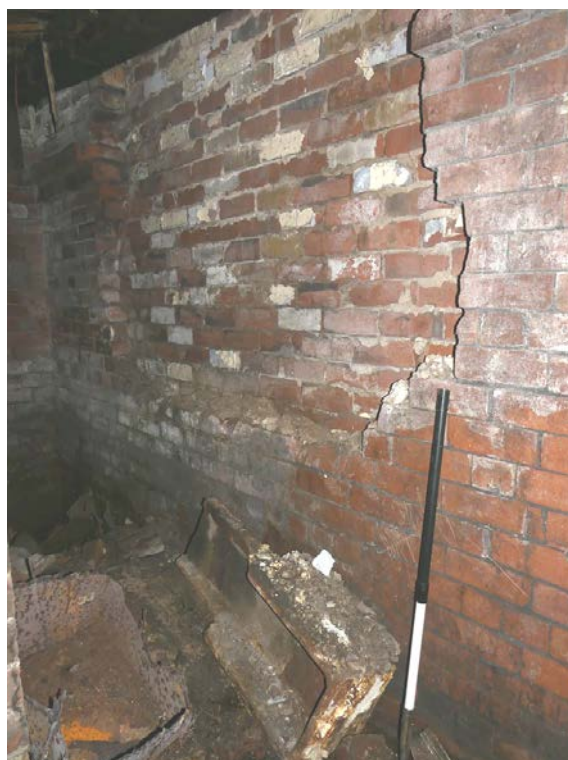
Plate 107: Ragged hole in the north-east elevation of the north-east end room (lower floor) of the mill building, Area D
