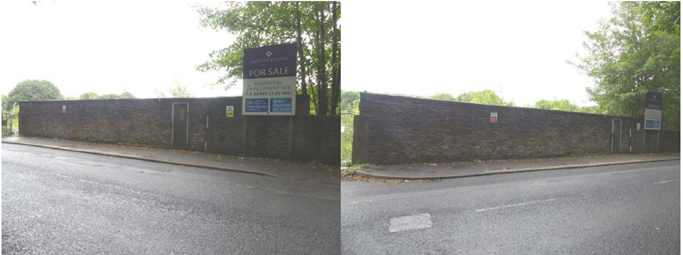
Plate 66 (left): North-west end of the south-west external elevation of the substation, Area C Plate 67 (right): South-east end of the south-west external elevation of the substation, Area C
