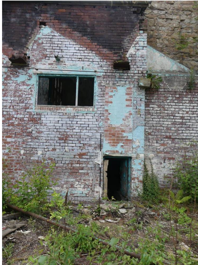
Plate 92: North-east doorway in the north-west external elevation of the mill building, Area D
