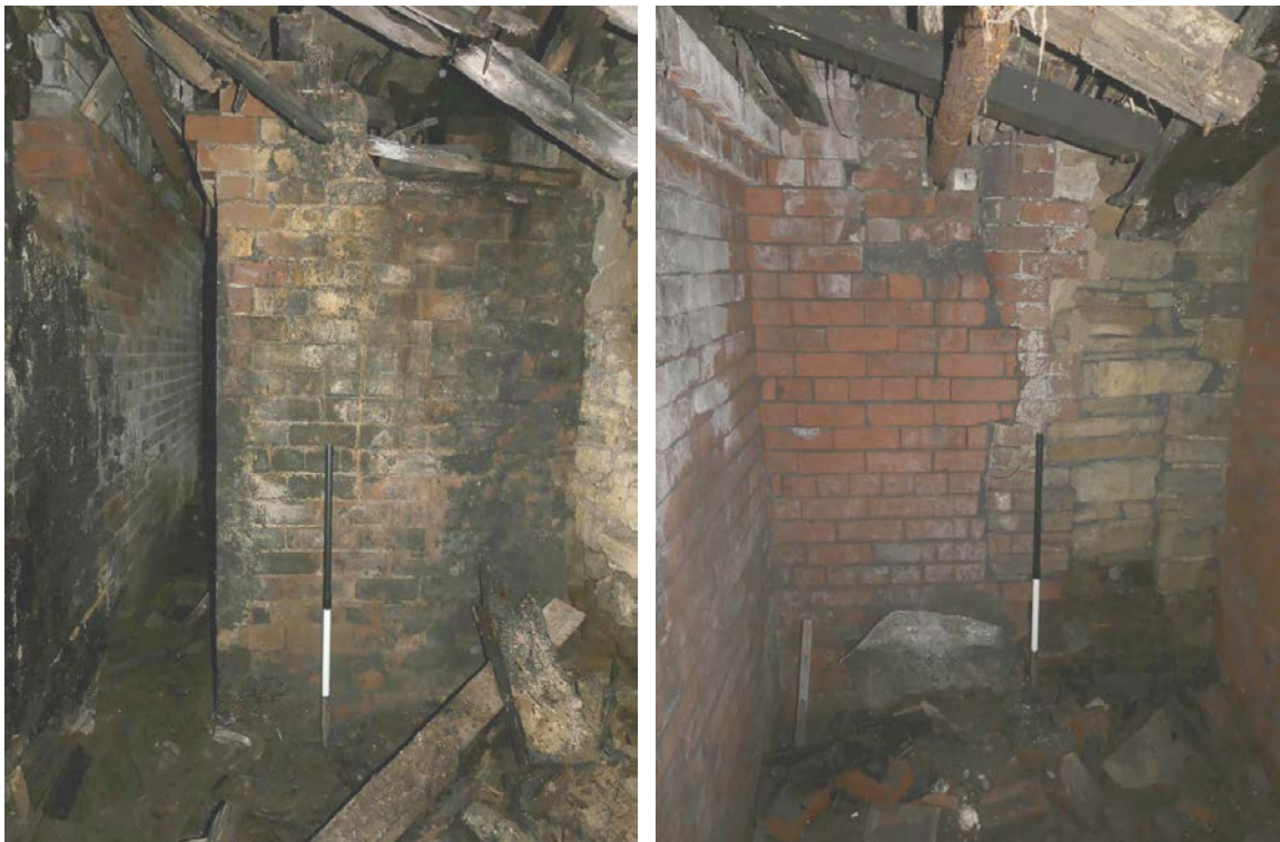
Plate 105 (left): Brick return at the north-east end of the south-east elevation of the north-east end room (lower floor) of the mill building, Area D
