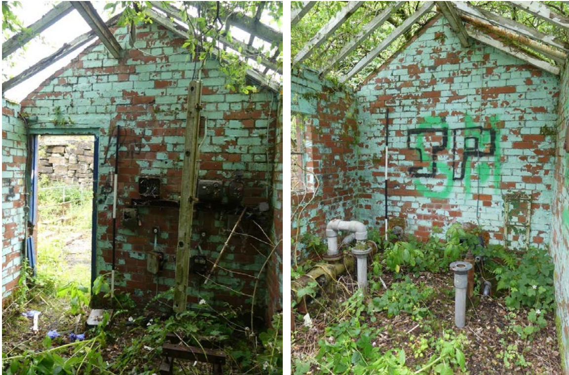
Plate 17 (left): Electrical boxes inside the small brick structure in Area A
