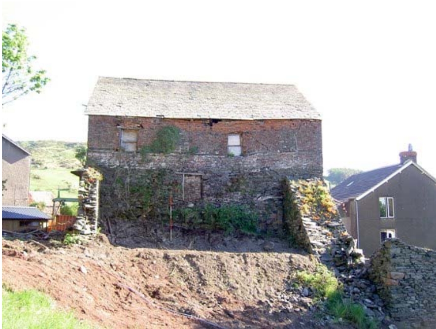
Plate 11: South external elevation after removal of scrub but prior to excavation of the wheel pit
