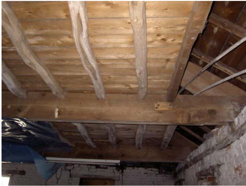
Plate 22: Typical beam and joists supporting floorboards on second floor. Note gouge in right side of beam
