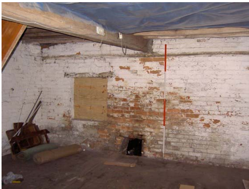
Plate 21: North elevation of second floor showing brick walling and chute at floor level into the north extension
