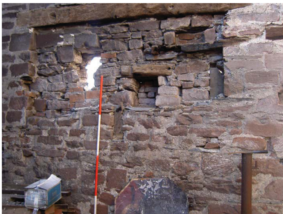
Plate 37: Blocked window and horse gin shaft housing in West wall of Building 9
