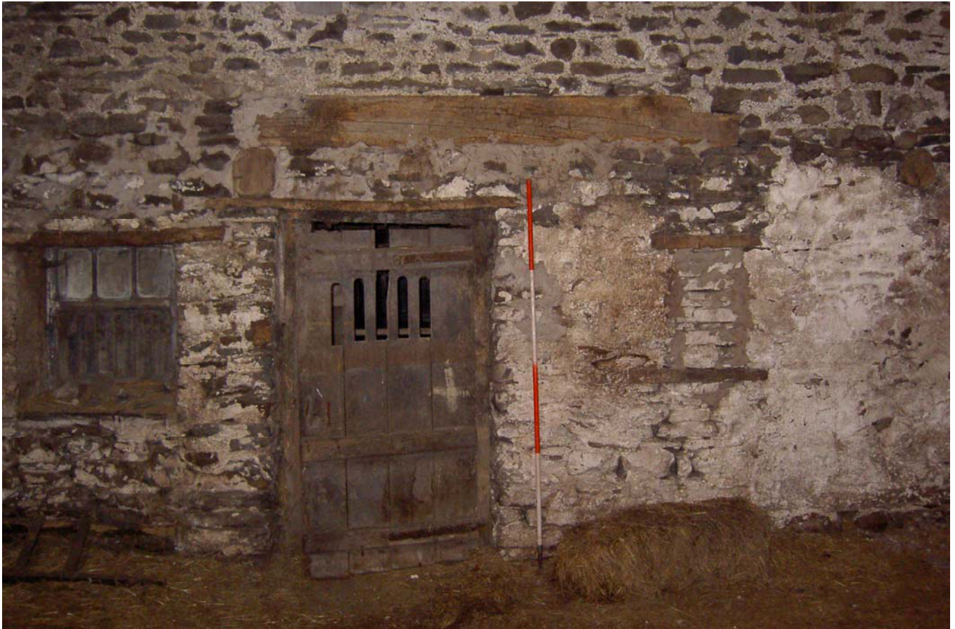
Plate 15: East end of north elevation, Room 1a, note sawn floor joist timbers for half loft
