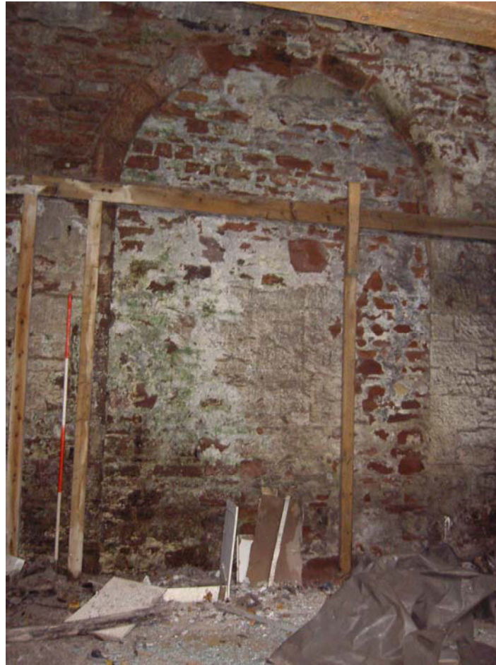
Plate 36: Blocked doorway at the west end of Building 3
