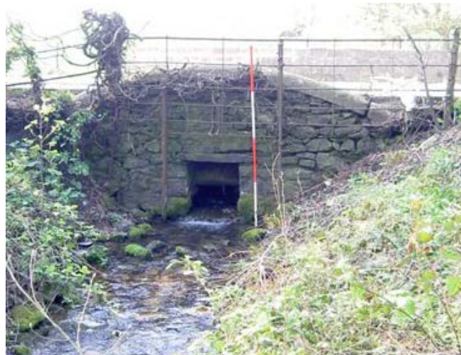
Plate 1: Culvert under the coast road at the north end of the estate (Site No. 101), looking west
