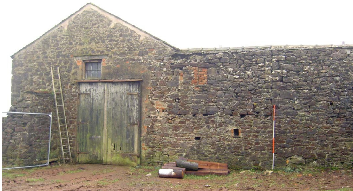
Plate 13: North elevation of Buildings 9, 8 and 7 (to the right of the ranging rod)
