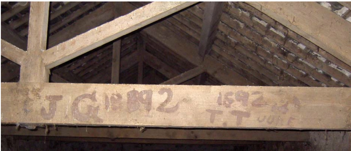
Plate 20: Graffiti on a truss in Building 2
